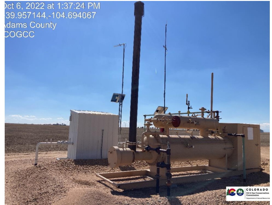
Pic 2 gas meter run, separator
