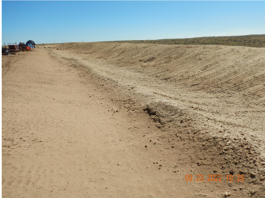
Photo 7. Photo taken from the southwestern location, facing East. Photo illustrates Operator has responded to the previous corrective action to comply with Rule 1002.c.
