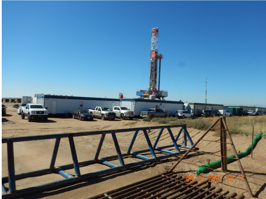
Photo 1. Photo taken from the east entrance of location, facing Southwest. Photo illustrates drilling operations are underway.
