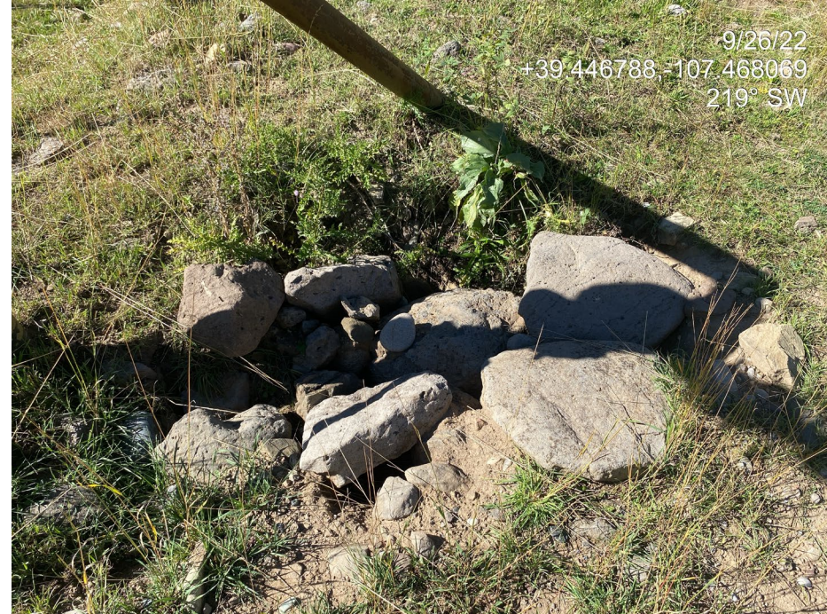
Photo 10. Photo shows a close-up of a hole/subsidence occurring at a rock drain.
