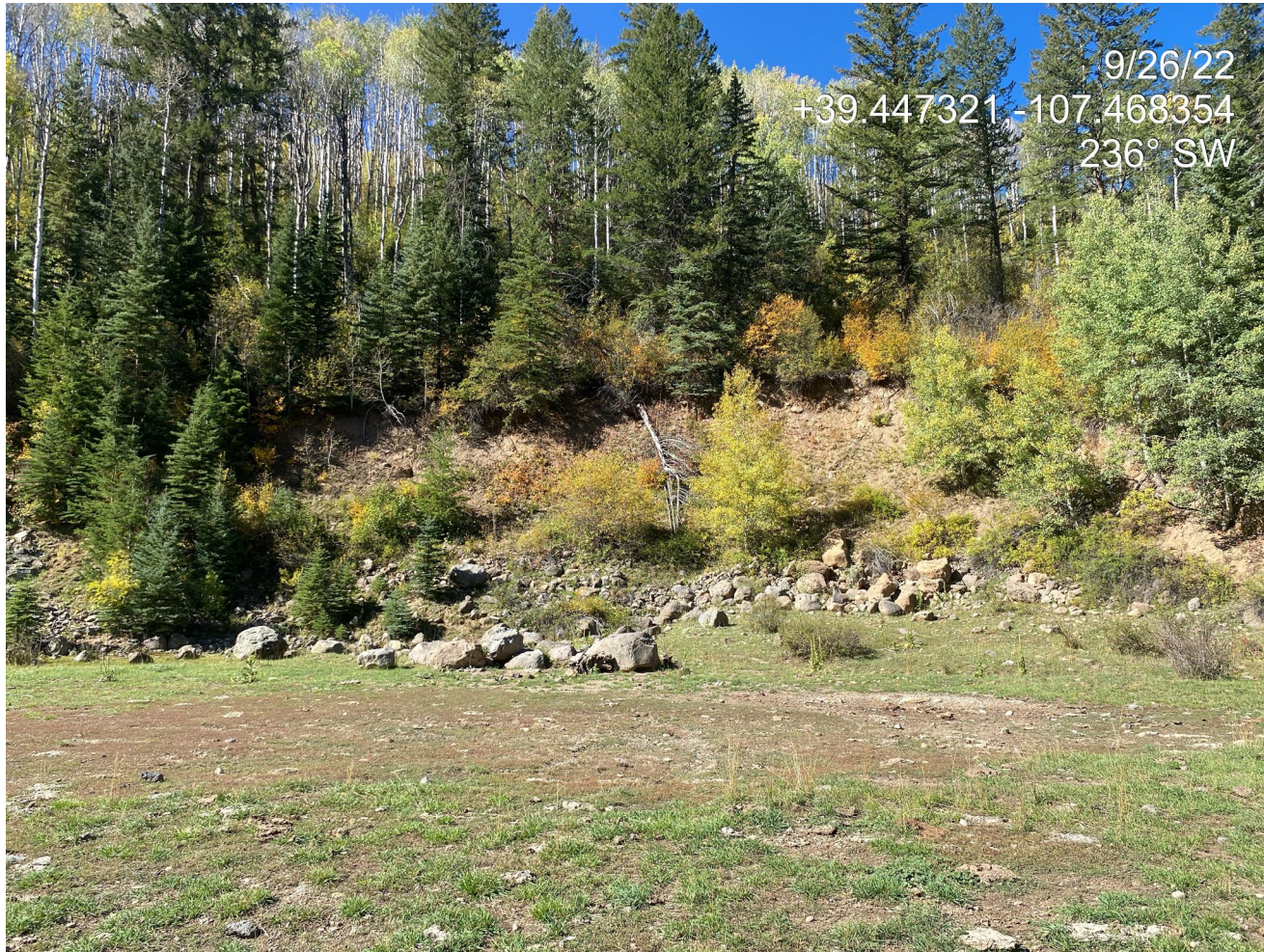
Photo 11. Photo taken from the north shows an overview of the eroding cut slope.
