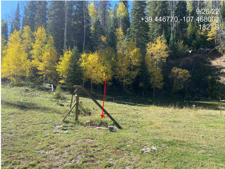
Photo 9. Photo shows where a hole/subsidence is occurring at a rock drain.
