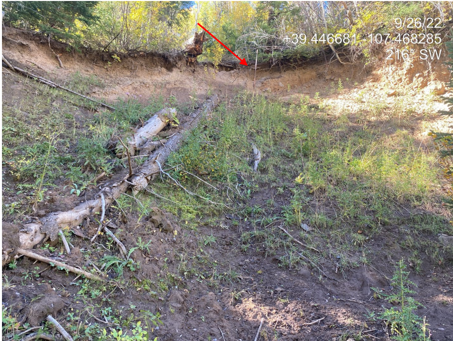
Photo 12. Photo taken from the southwest of the Location shows the cut slope is eroding and undercutting into undisturbed areas above the cut exposing roots. Arrow indicates an undermined fence. Vegetation at the center of the cut is Canada thistle (List B Noxious). Note also pedestals around vegetation throughout slope.
