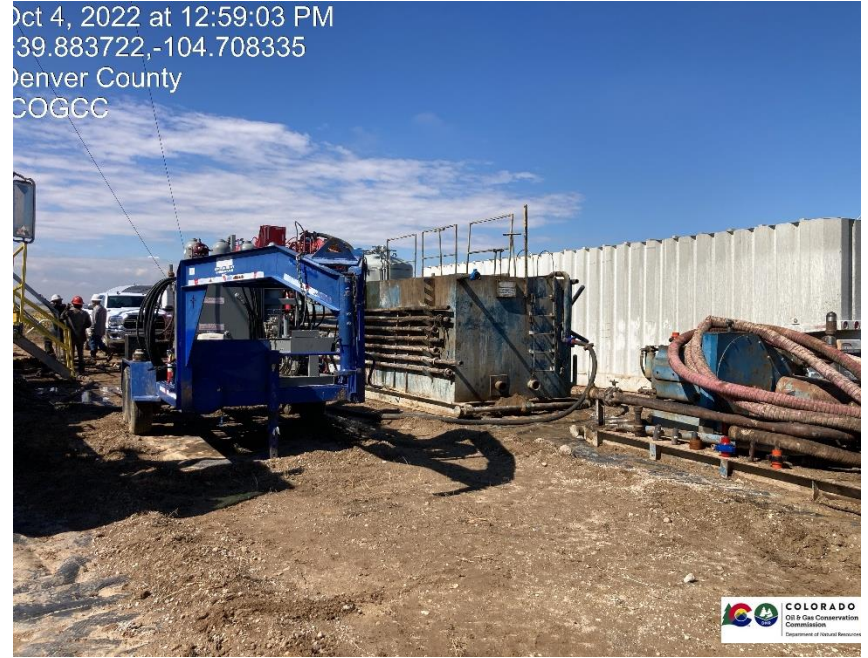
Pic 2 Pump, tank, accumulator
