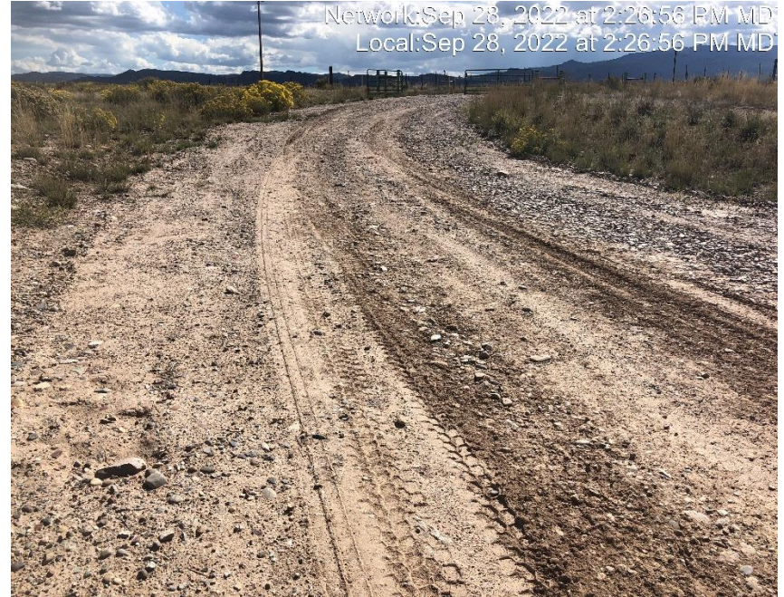
Photo #7850 Insufficient tracking BMP at entrance to location
