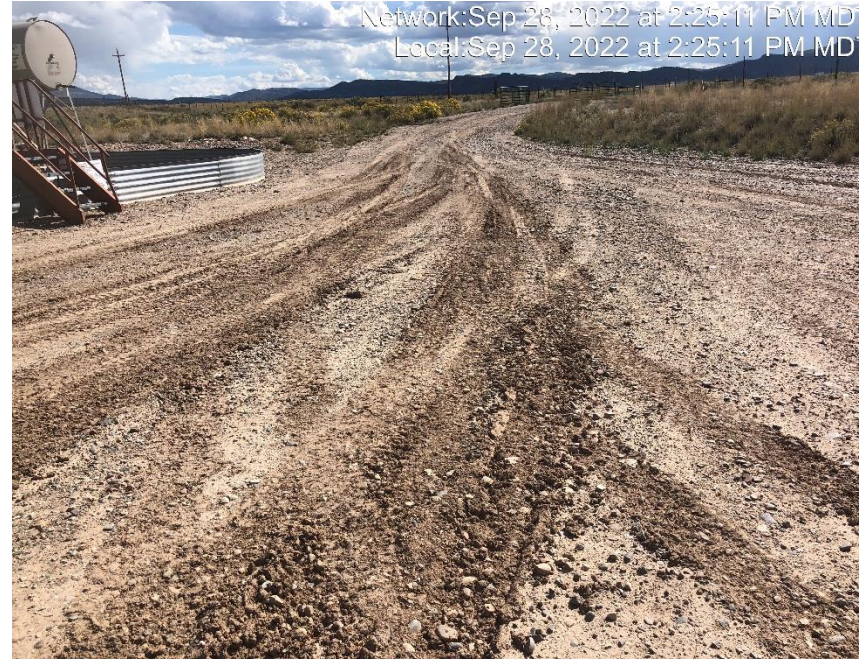
Photo #7846 Location lacks stabilization.
