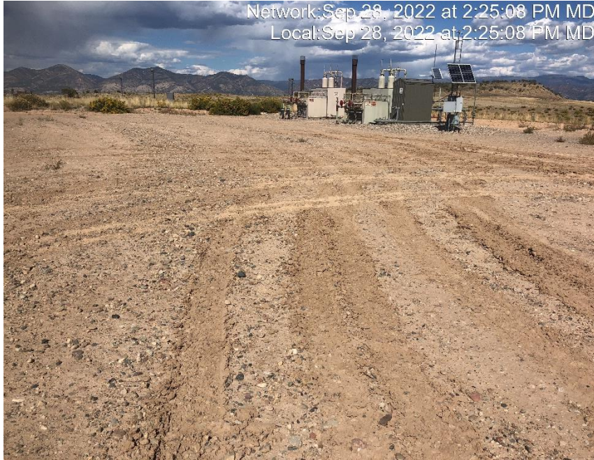
Photo #7845 Location lacks stabilization.
