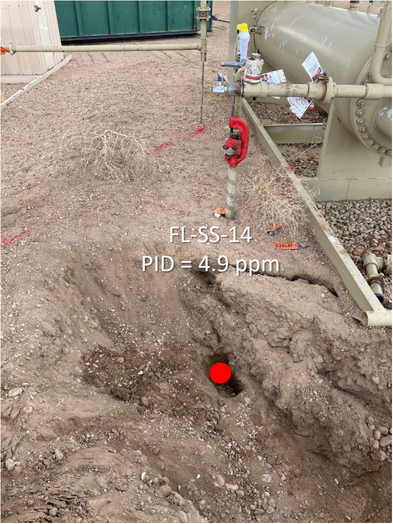
Looking north Pt B. / terminus at separator sampled for lab No petroleum hydrocarbon staining or odor observed
