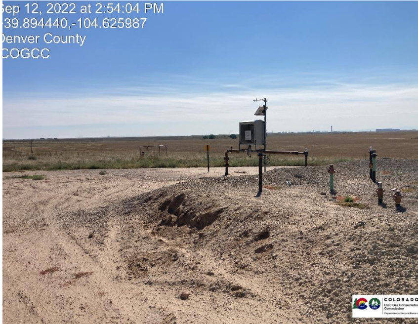
Pic 3 Gas Meter Run
