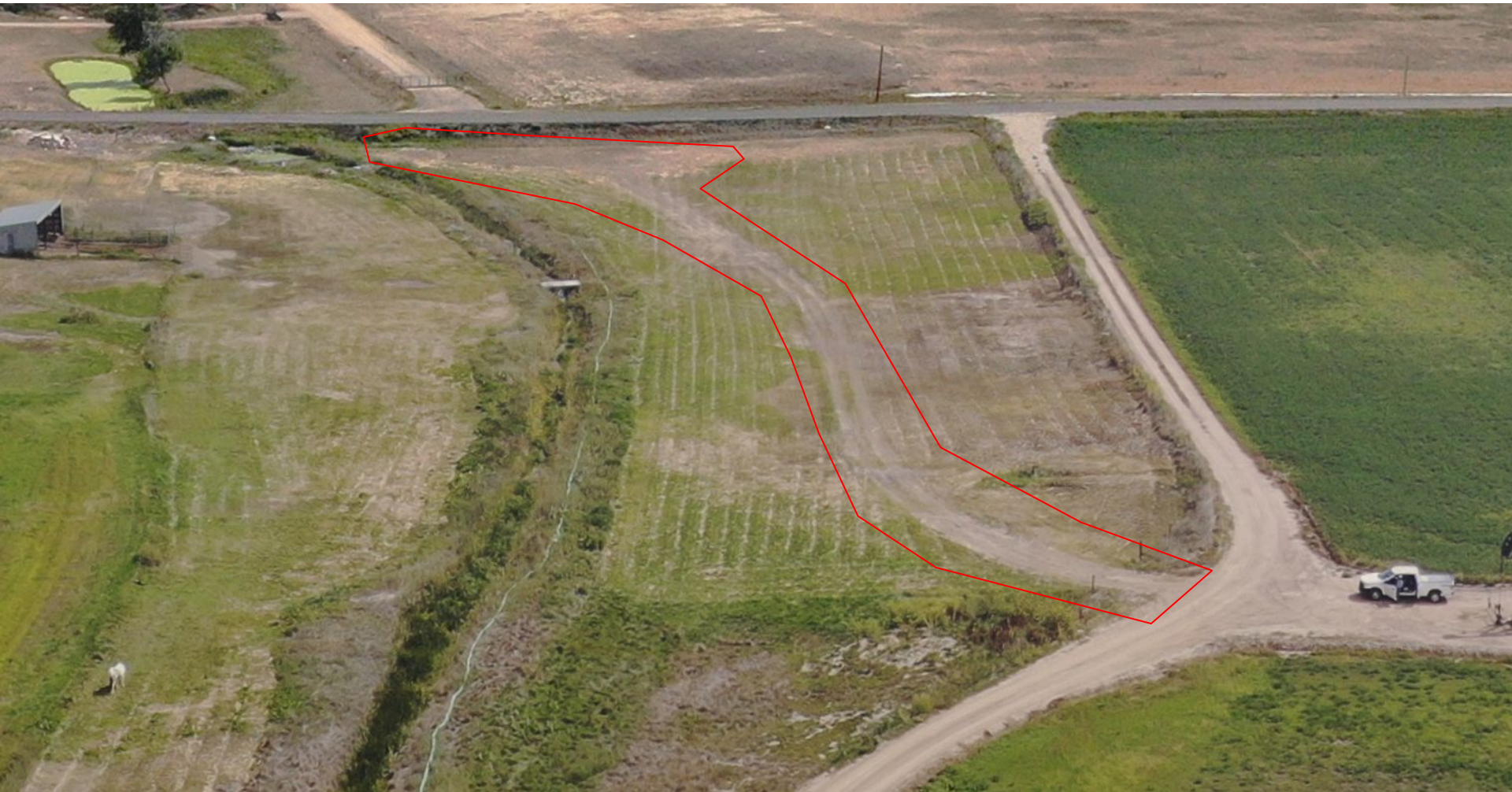
Photo 1. COGCC drone aerial imagery taken on September 13, 2022 documenting the scope of reclamation work to be performed. This image is the approximate extent of reclamation along the eastern project area.
