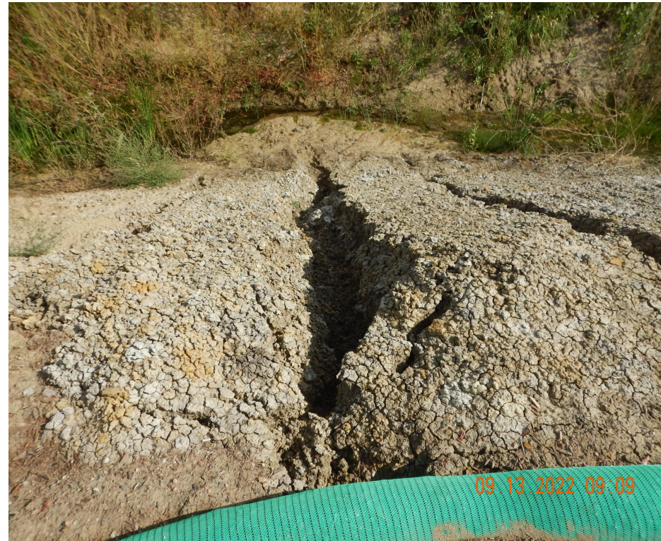
Photo 7. Photo taken from the western fill slope, facing North. Photo illustrates erosion along the fill slope that needs to be repaired during reclamation. The erosion is believed to be from a recent irrigation event by the surface owner.
