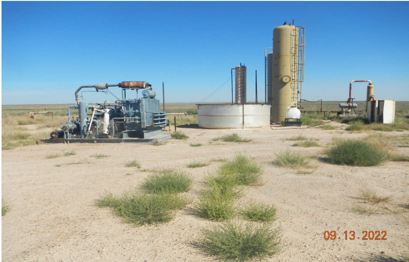
Photo 1. Facing northeast toward the gas treatment facility.
