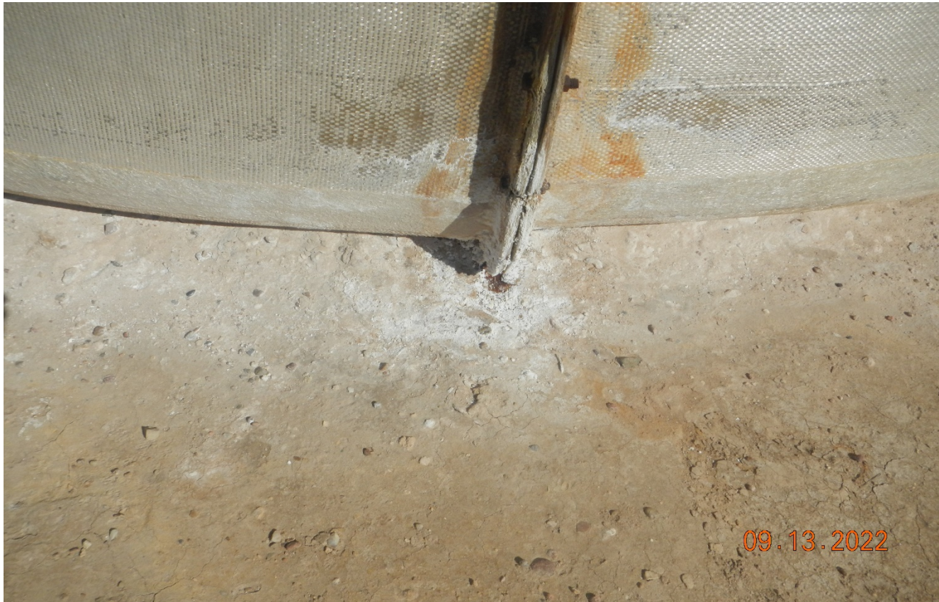
Photo 11. There are signs of a previous leak at the tanks due to white stained soils at the base of the tanks.
