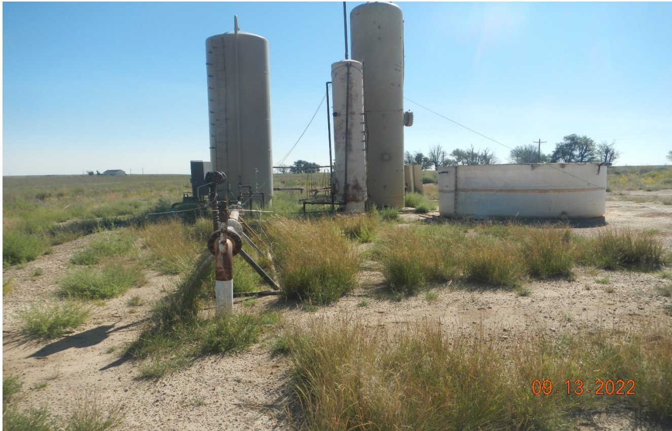
Photo 14. Facing east toward the facility. There are weeds and vegetation around the equipment which is a fire hazard.
