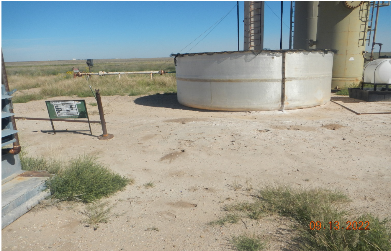
Photo 4. Facing toward the open top tank. It appears the tank has previously leaked due to white stained soil. There is no secondary containment around the tank. There is no signage on the tank. Previous corrective action is not completed.
