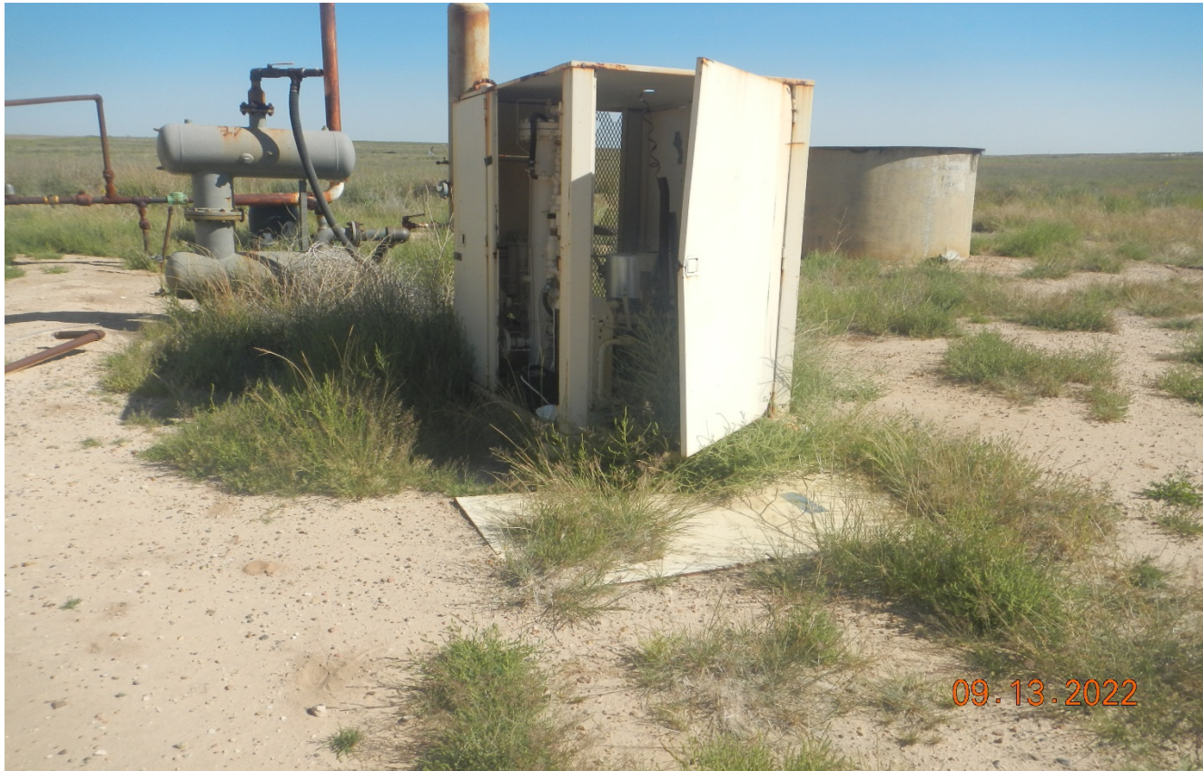
Photo 6. There is equipment not maintained on location. Door has fallen off this shed. Previous corrective action is not completed.
