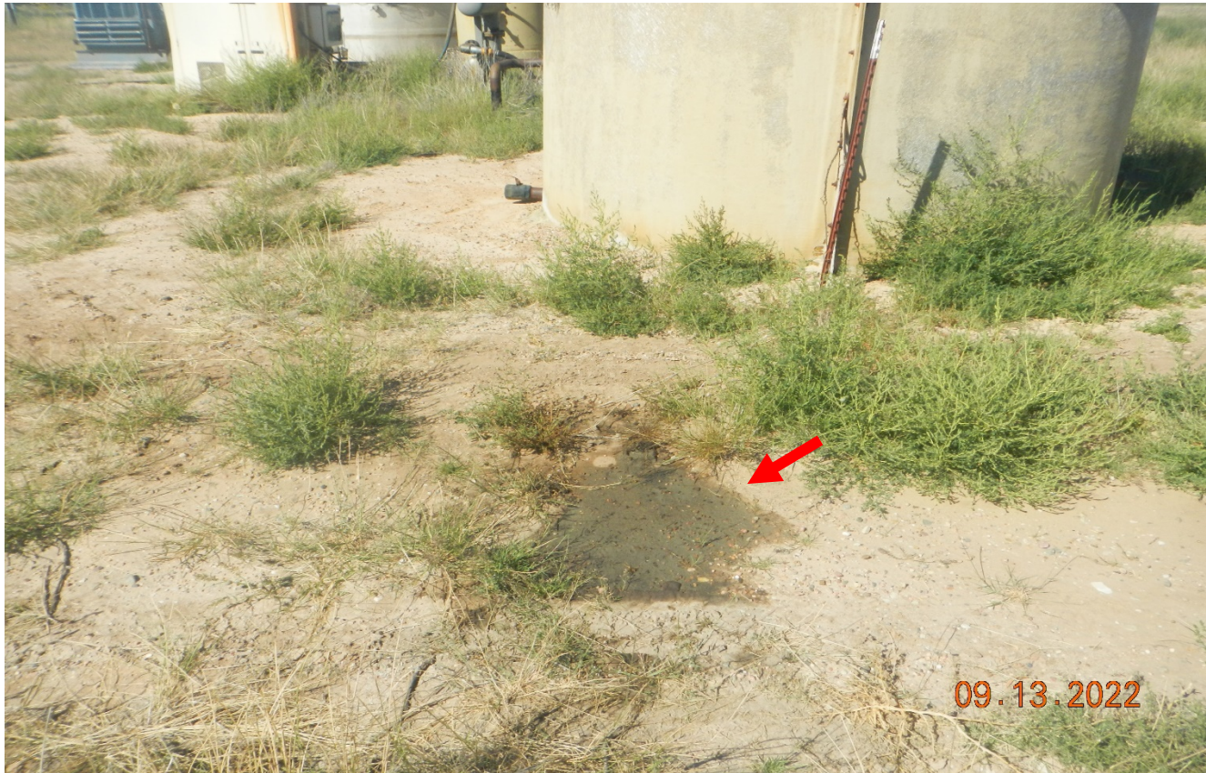
Photo 9. There is oily stained soil at red arrow which appears to be fluids which were drained from the tank. Stained soil need to be cleaned up and properly disposed.
