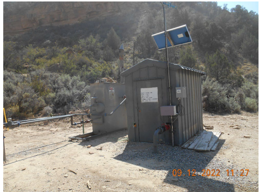
Separator and Meter housing
