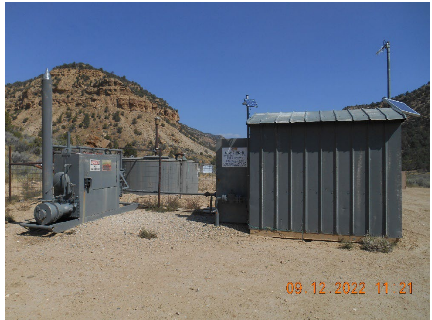
Separator and Meter housing
