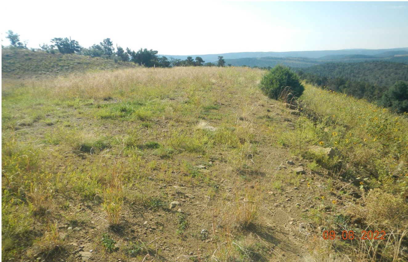
Photo 2. Facing toward the west fill slope at the location. The vegetation appears to be stabilizing this area.
