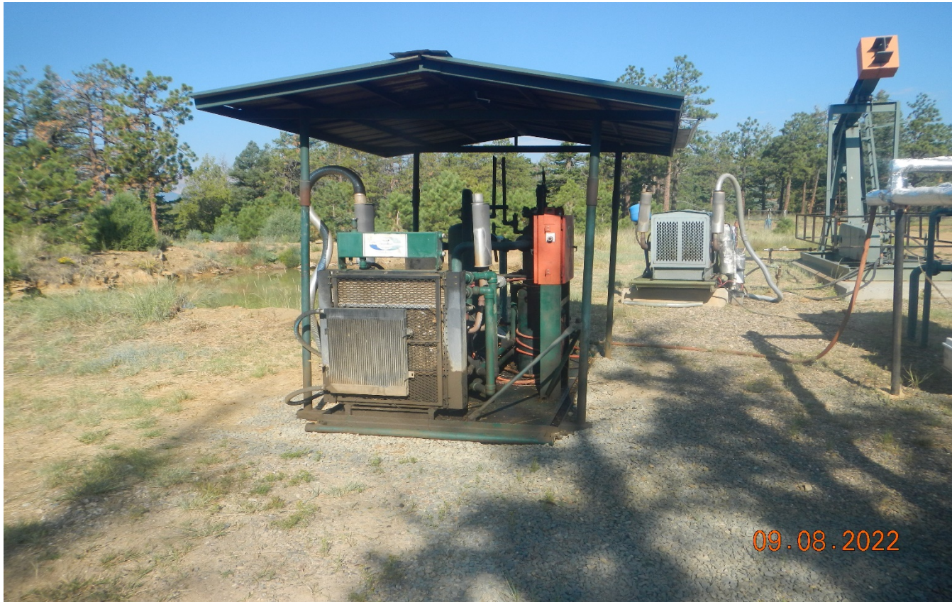
Photo 2. Stained soils near the engine skid have been cleaned up.
