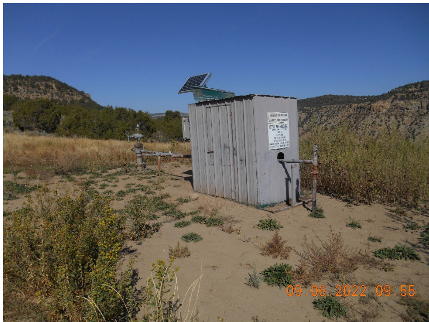
Wellhead and Meter housing
