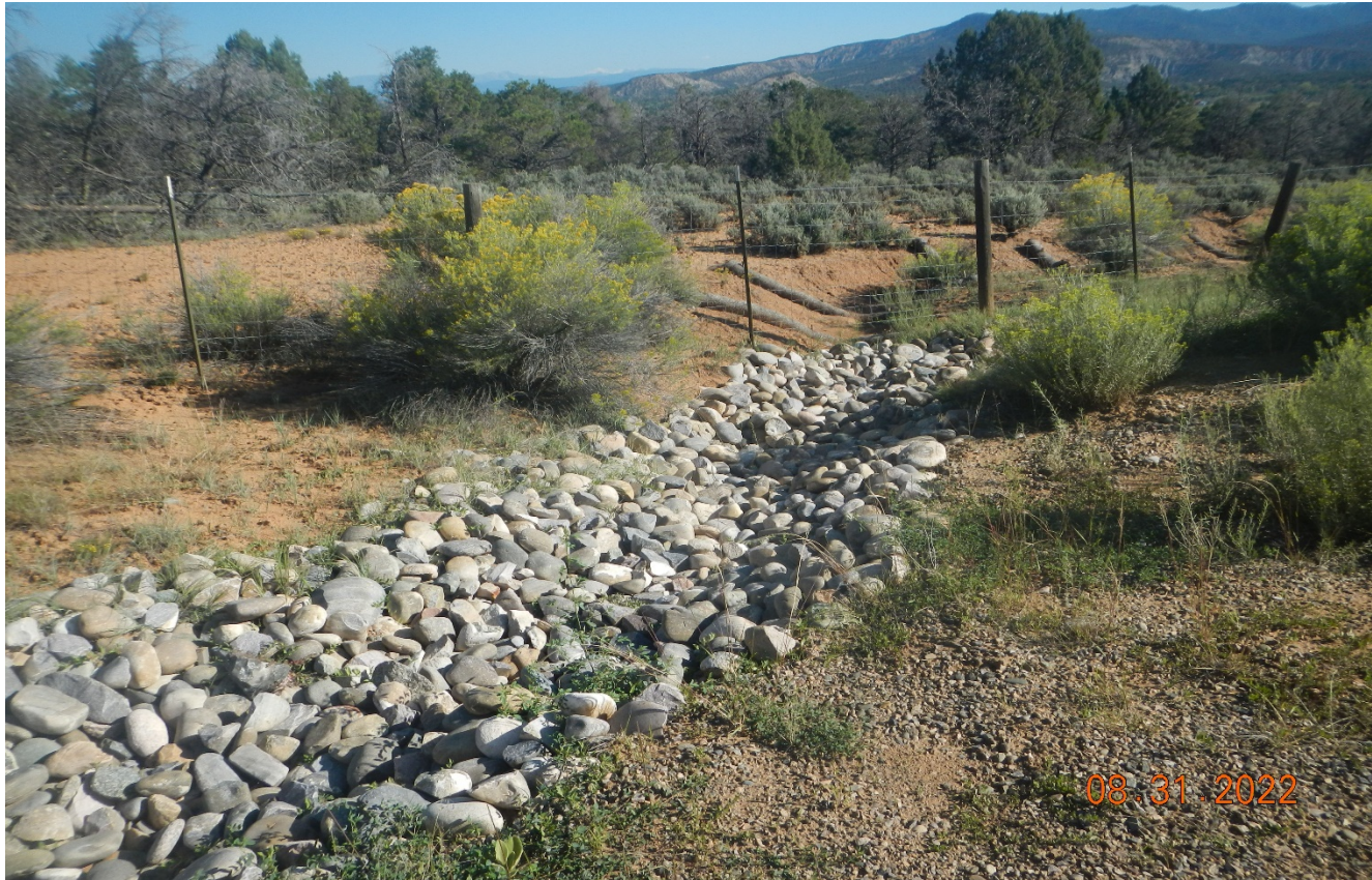
Photo 2. Northwest side of the location. There has been rock rip/rap installed in the erosion gully that was cited in the previous inspection.
