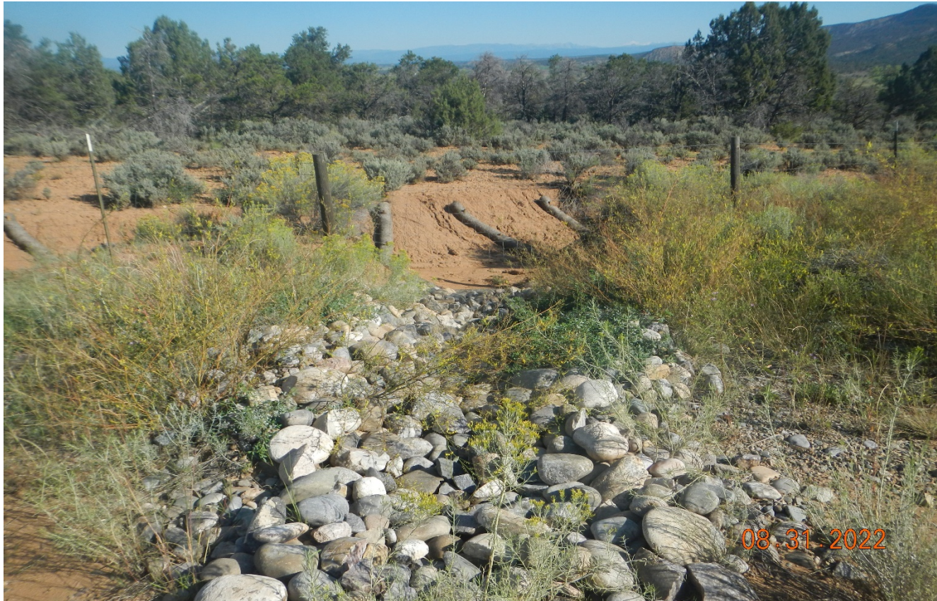
Photo 3. There are wattles and rock rip/rap installed at the northwest side of the location.
