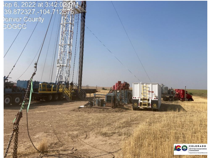
Pic 2 tanks / pump
