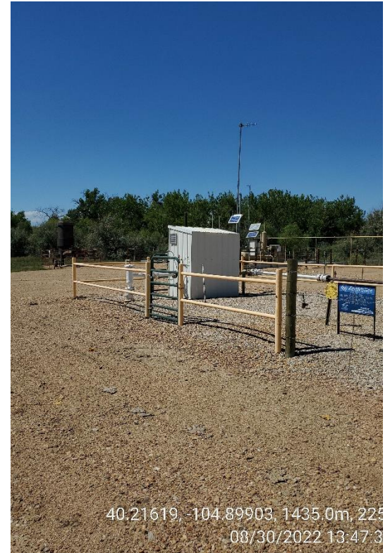
Photo 3 GMR and Pig Station.
