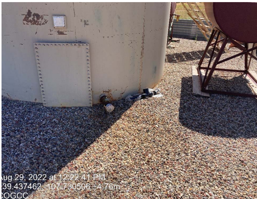
Valve on ground/stored supply
