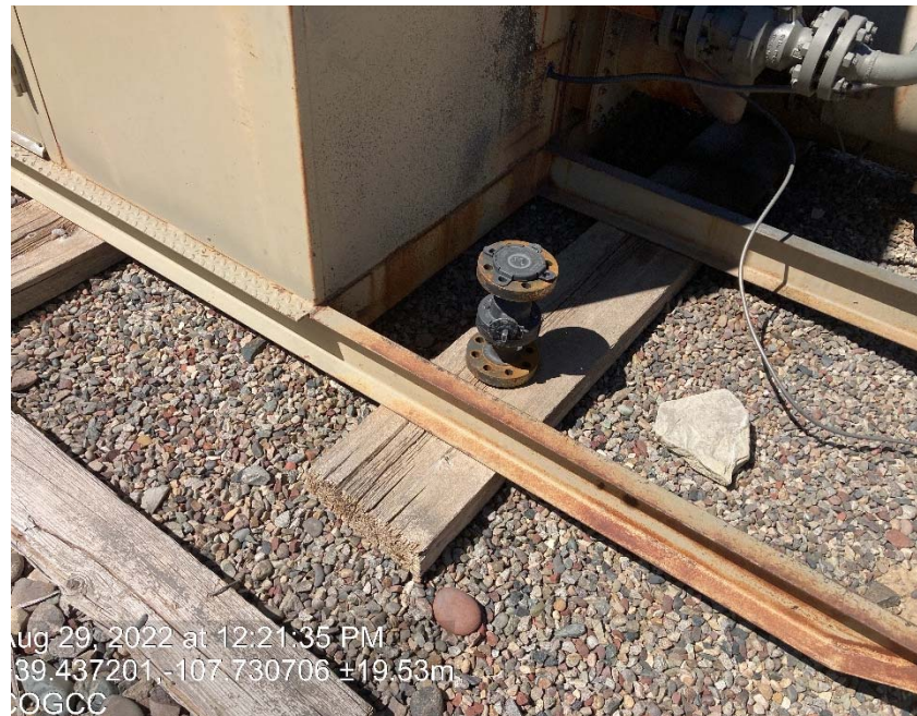
Valve on ground/stored supply
