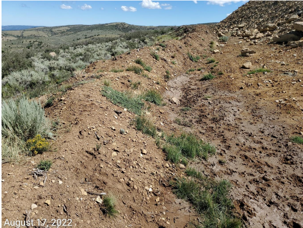
Photo 7: Photo taken from the west end of the Location. Photo shows topsoil stockpile in use as part of the stormwater sediment trap/basin. Photo shows evidence of stormwater runoff, ponding, and sediment transport/deposition along the stockpiles. Photo also example showing topsoil stockpiles remain bare/exposed soil; BMPs to protect soils remain missing or insufficient.
