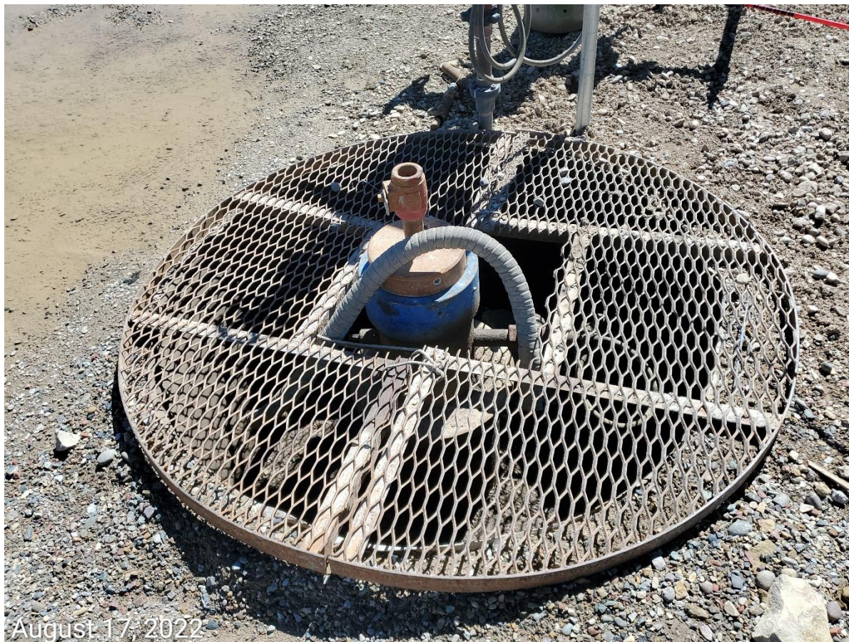
Photo 19: Photo shows pipe/cellar/conductor/equipment remains evident a the PA'd ELU J14 FED #11B-14-496 well site
