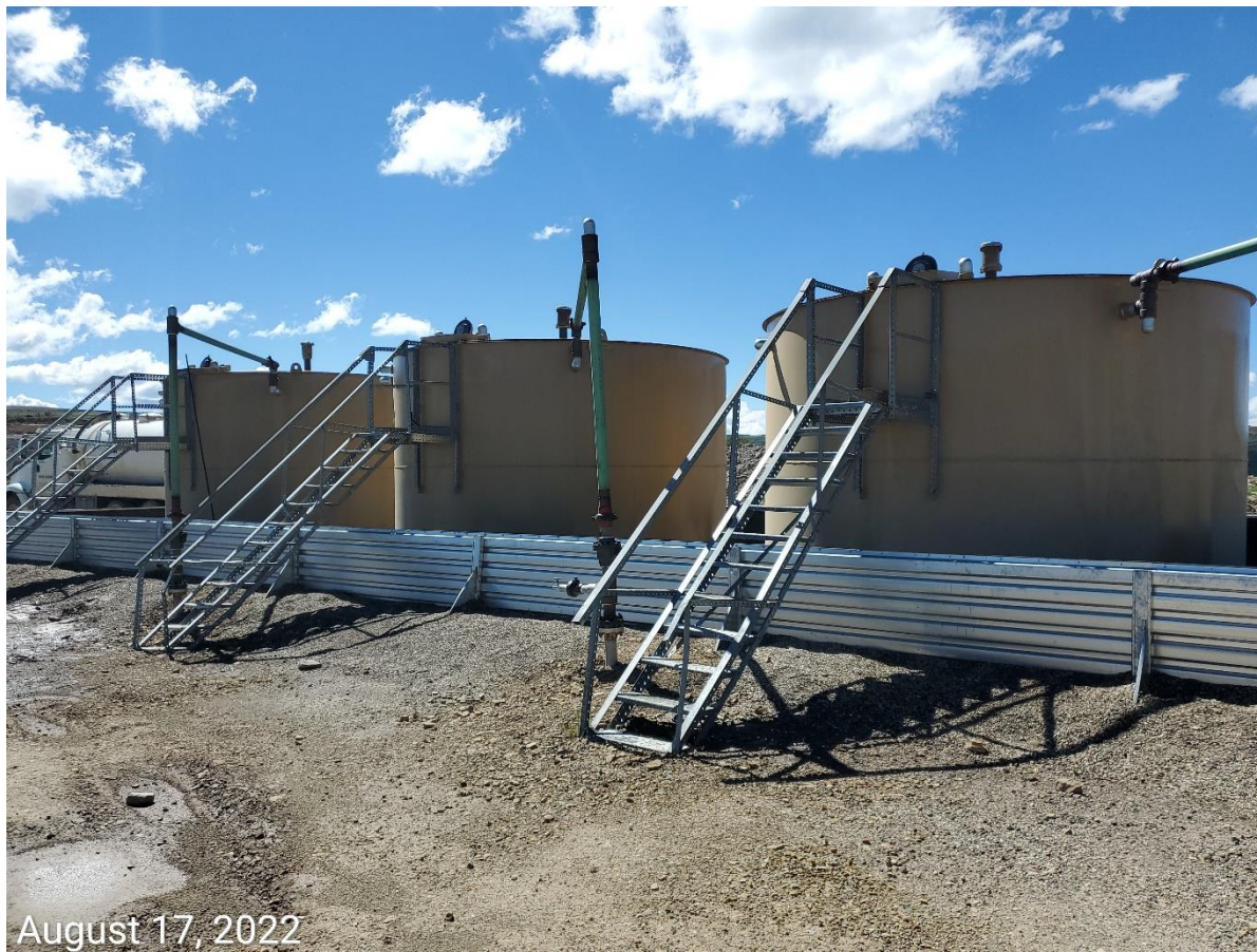
Photo 17: Photo taken from the tank battery on the southwest end of the Location. Photo shows signage and labeling remain missing from the tanks/battery.
