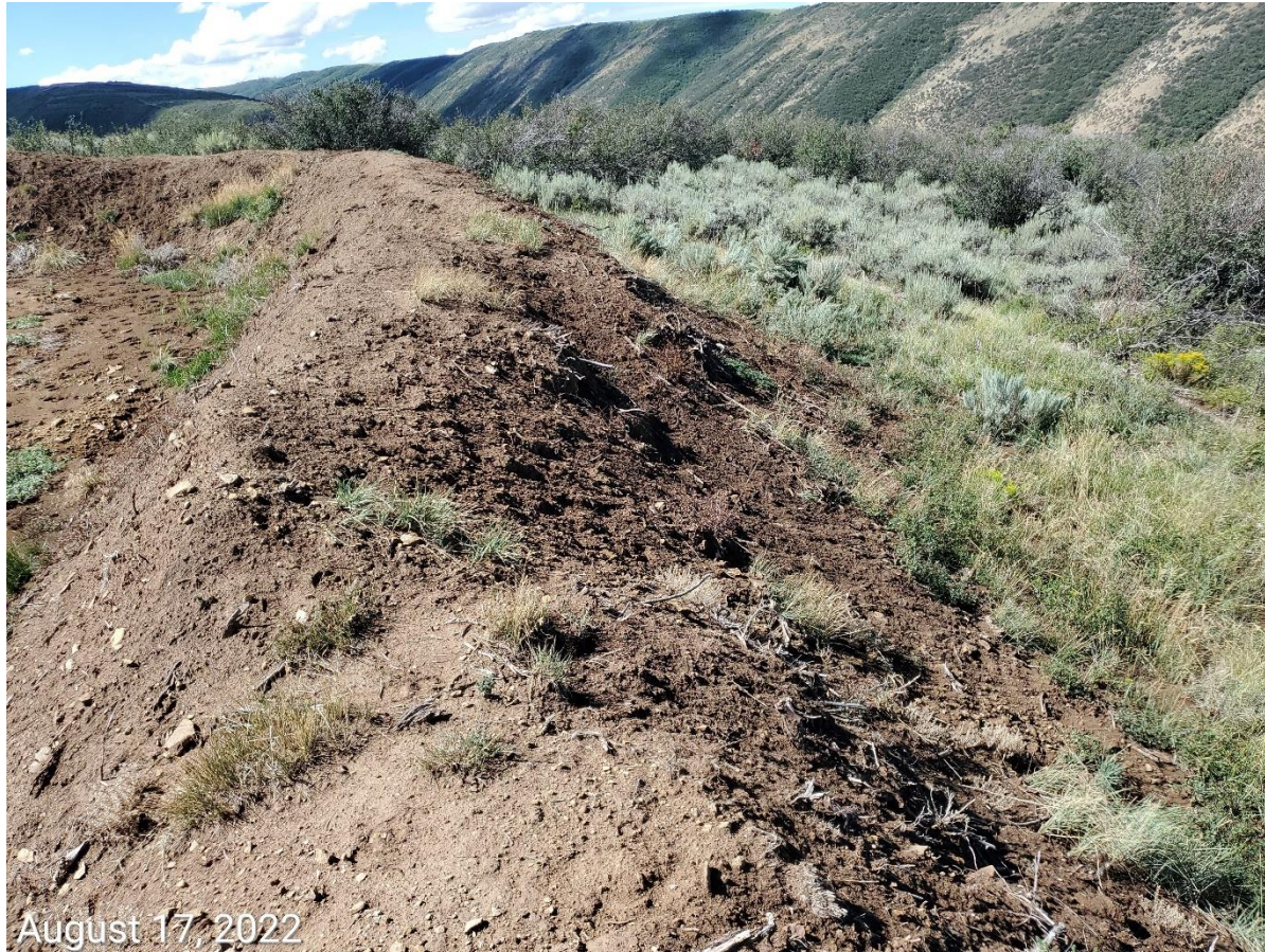
Photo 10: Photo example showing topsoil stockpiles along perimeter of the Location remain bare and exposed; BMPs to protect topsoil remains missing or insufficient; erosion degradation evident.
