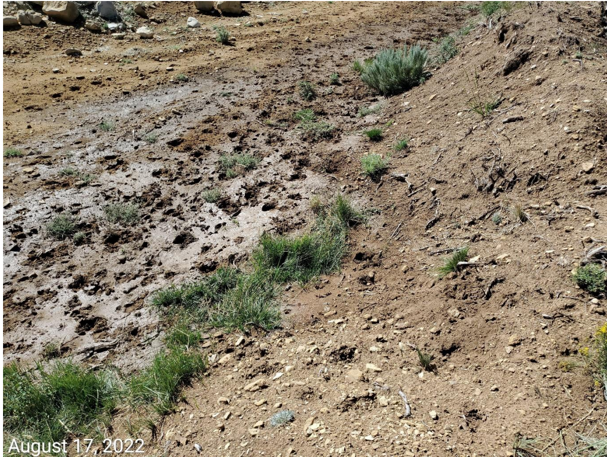
Photo 6: Photo taken from the west end of the Location. Photo shows topsoil stockpile in use as part of the stormwater sediment trap/basin. Photo shows evidence of stormwater runoff, ponding, and sediment transport/deposition along the stockpiles. Photo also example showing topsoil stockpiles remain bare/exposed soil; BMPs to protect soils remain missing or insufficient.
