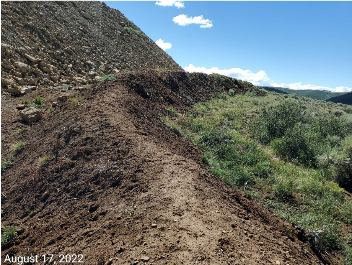
Photo 11: Photo example showing topsoil stockpiles along perimeter of the Location remain bare and exposed; BMPs to protect topsoil remains missing or insufficient; erosion degradation evident.
