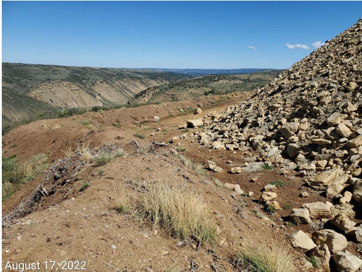
Photo 13: Photo example showing the topsoil stockpile in use as part of the perimeter stormwater ditch/berm and sediment trap/basin. Photo also example soils remain bare; BMPs to protect soils remain missing or insufficient.
