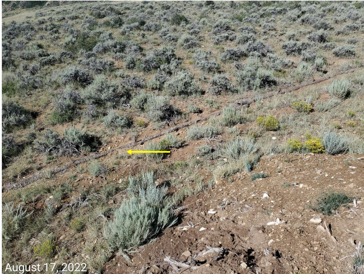
Photo 14: Photo example showing a single row of straw wattle erosion log in place along perimeter of the Location. BMP appears to have exceeded its manufactured life span and does not appear to be maintained; wattle in disrepair along sections; offsite sediment transport and deposition on top of wattles apparent (arrow).
