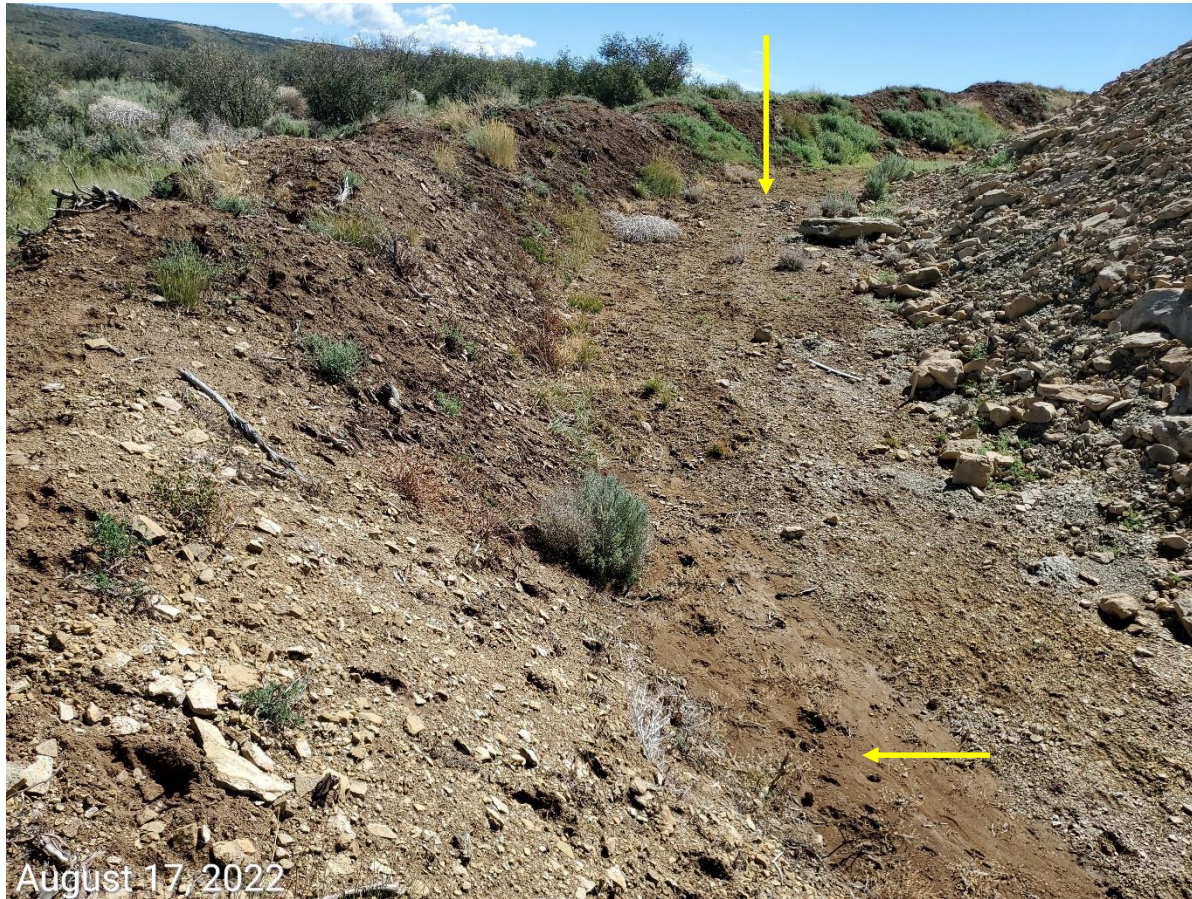
Photo 4: Photo example showing the topsoil stockpile in use as part of the perimeter stormwater ditch/berm. Photo also shows water movement patterns due to stormwater runoff (arrow) that has resulted in sediment transport, deposition (red arrow) and ponding along the stockpile. Photo also example showing soils at the stockpile remain bare; BMPs to protect soils remain missing or insufficient.
