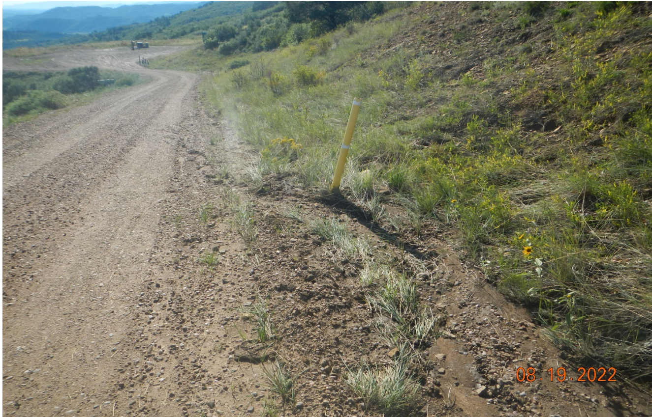
Photo 2. It appears stormwater is going around the culvert. This area should be shoveled out to direct stormwater toward the culvert.
