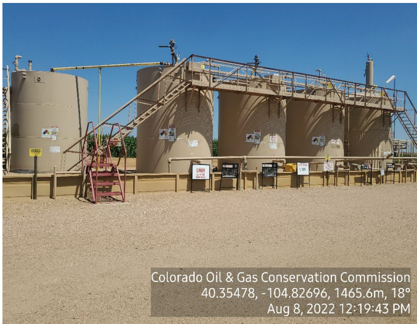
Photo 5: Centralized Tank Battery
