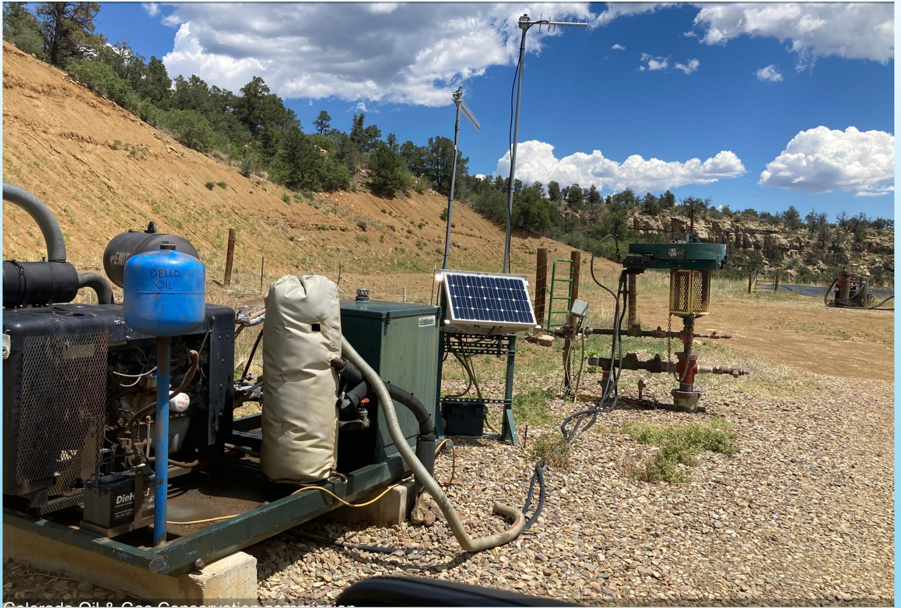
PHOTO 3: V WELLHEAD AND EQUIPMENT
