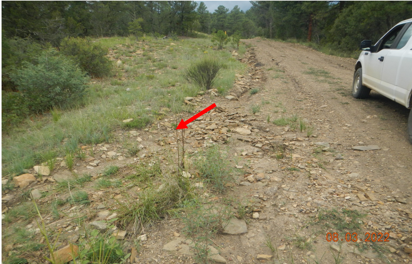
Photo 3. Stormwater should be directed off the road instead it appears to be going down the road causing erosion shown in previous photo.
