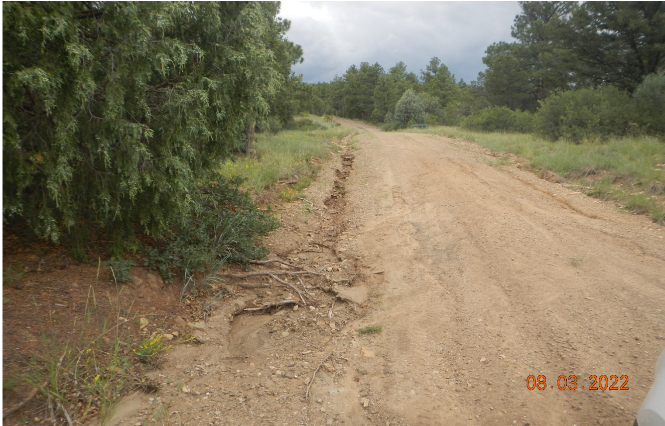
Photo 2. Further along the road there is erosion channeling occurring on the roadside. BMP's need to be installed to prevent erosion.
