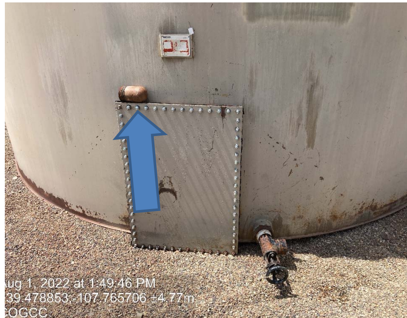
Valve on tank missing cap/plug
