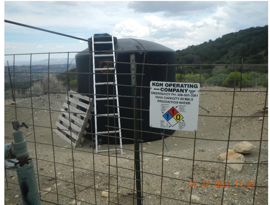
No tank battery sign.
