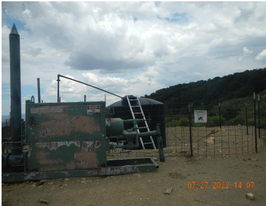
No tank battery sign.
