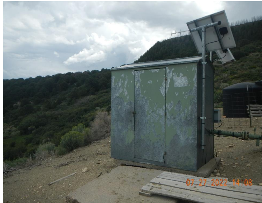
No tank battery sign.
