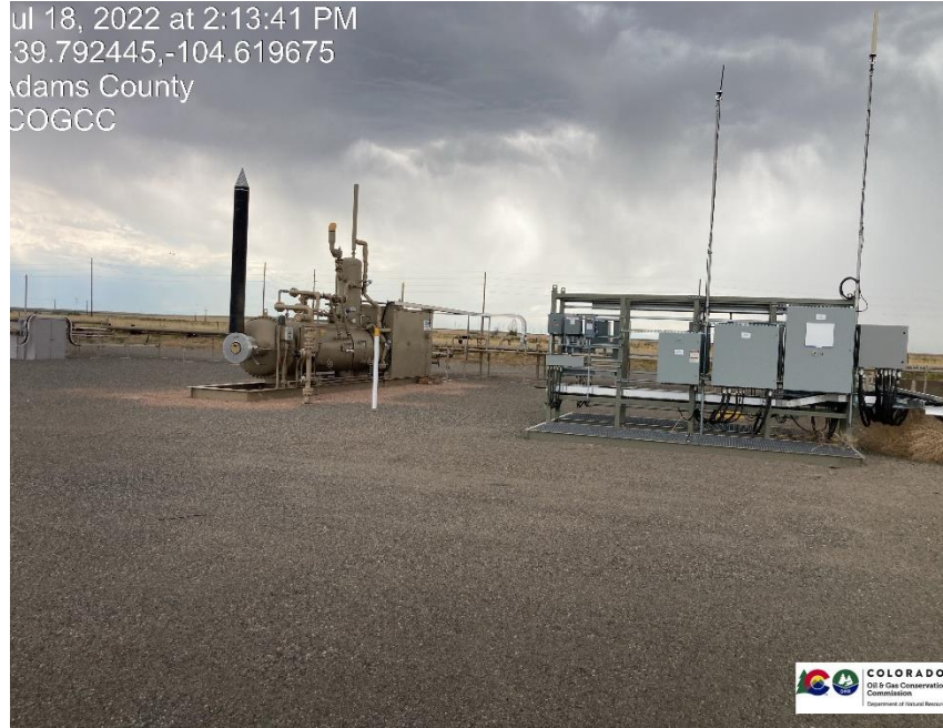
Pic 3 Electric equipment / Separator
