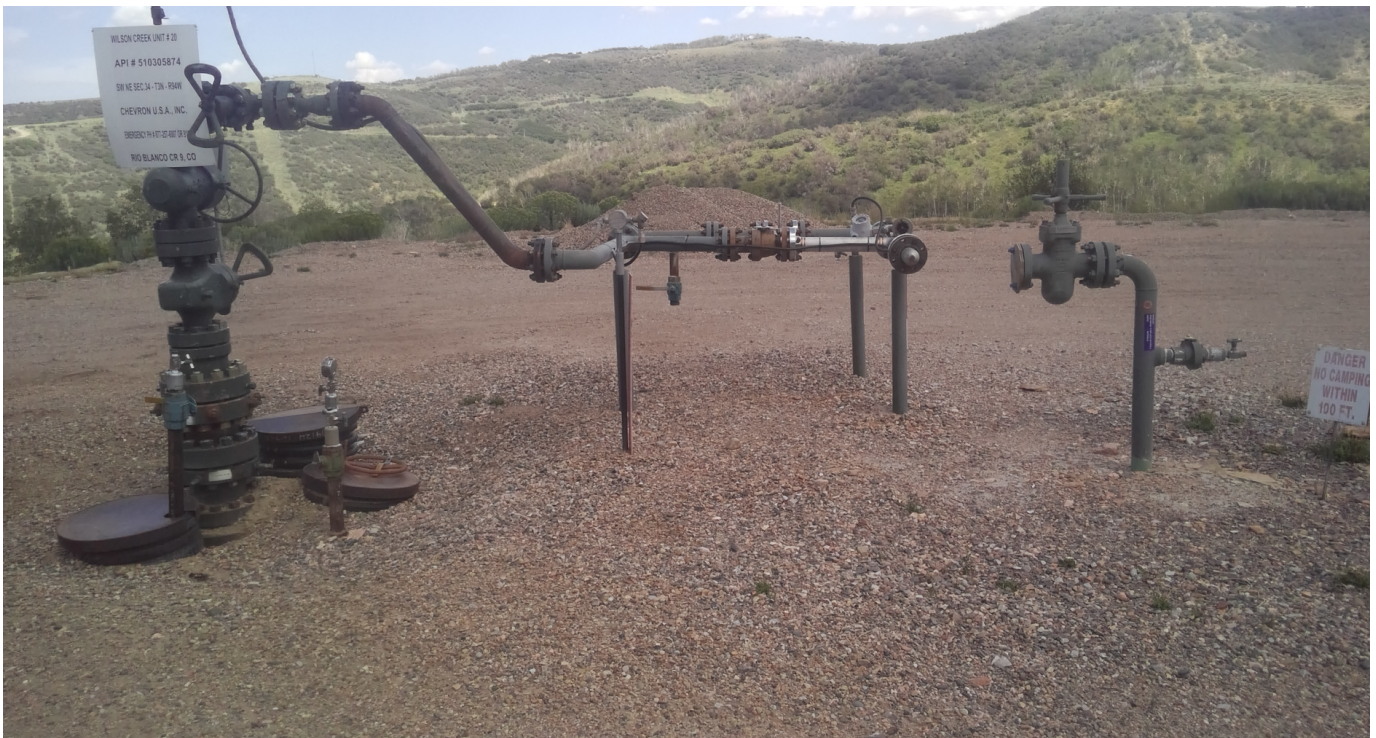
CA2: Debris has been removed
