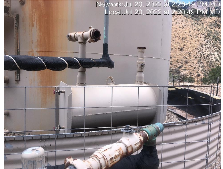
Photo #7219 Multiple places with unused equipment.
