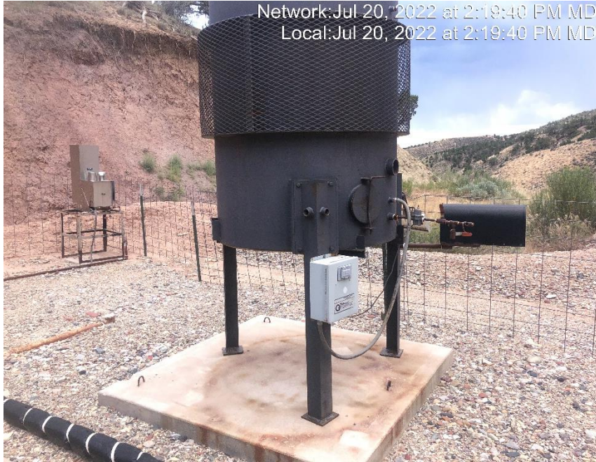
Photo #7216 Multiple places with unused equipment.
