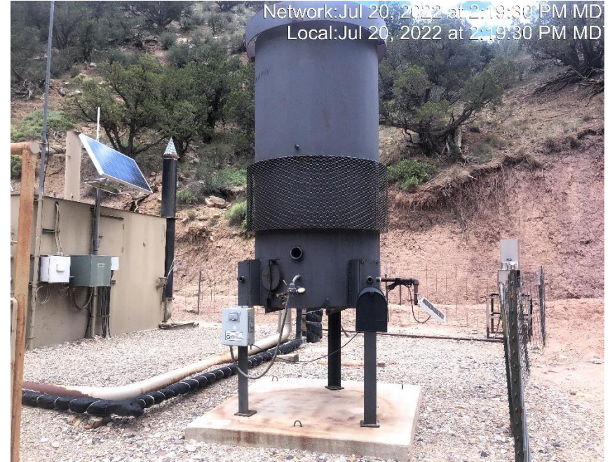
Photo #7215 Multiple places with unused equipment.
