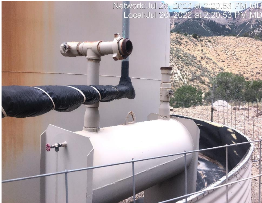
Photo #7220 Multiple places with unused equipment.
