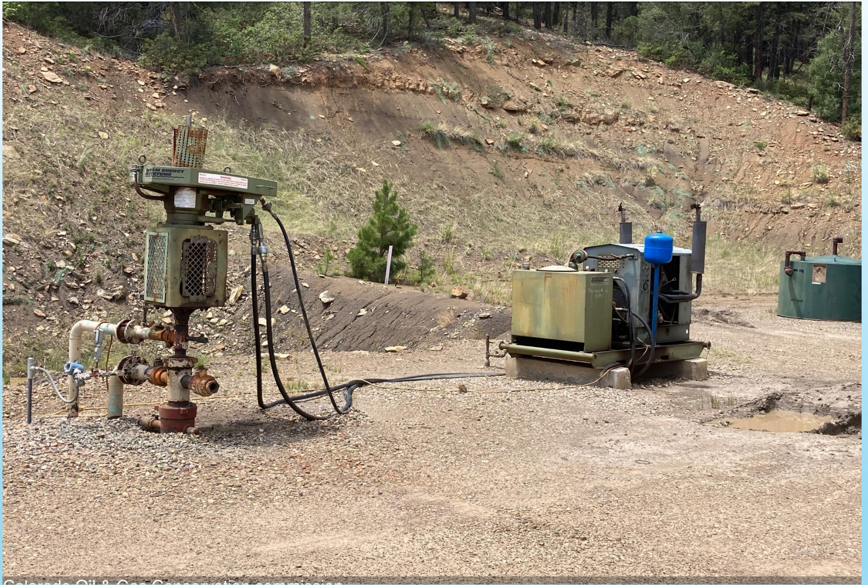
PHOTO 3: WELLHEAD AND EQUIPMENT
