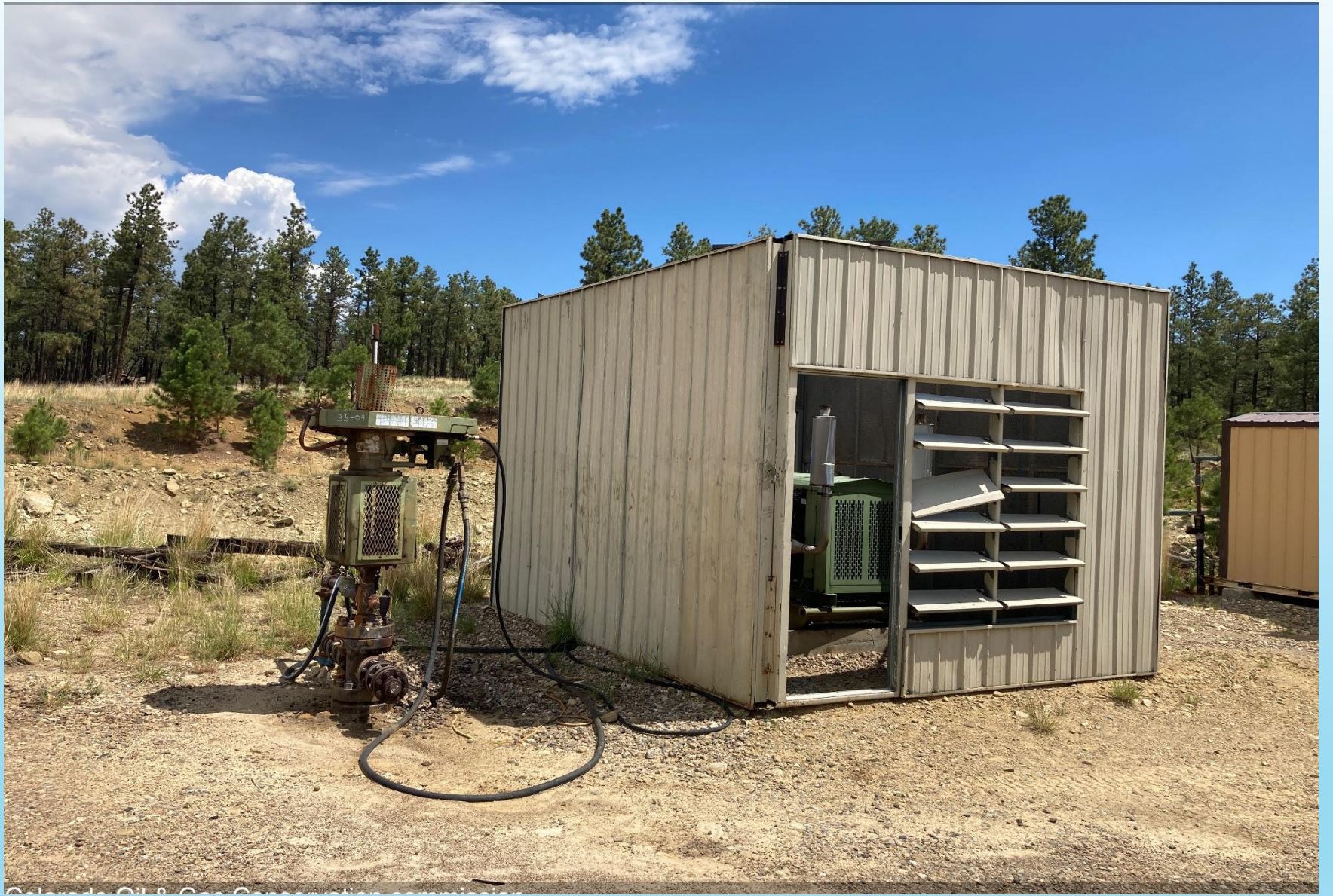
PHOTO 3: WELLHEAD AND EQUIPMENT
