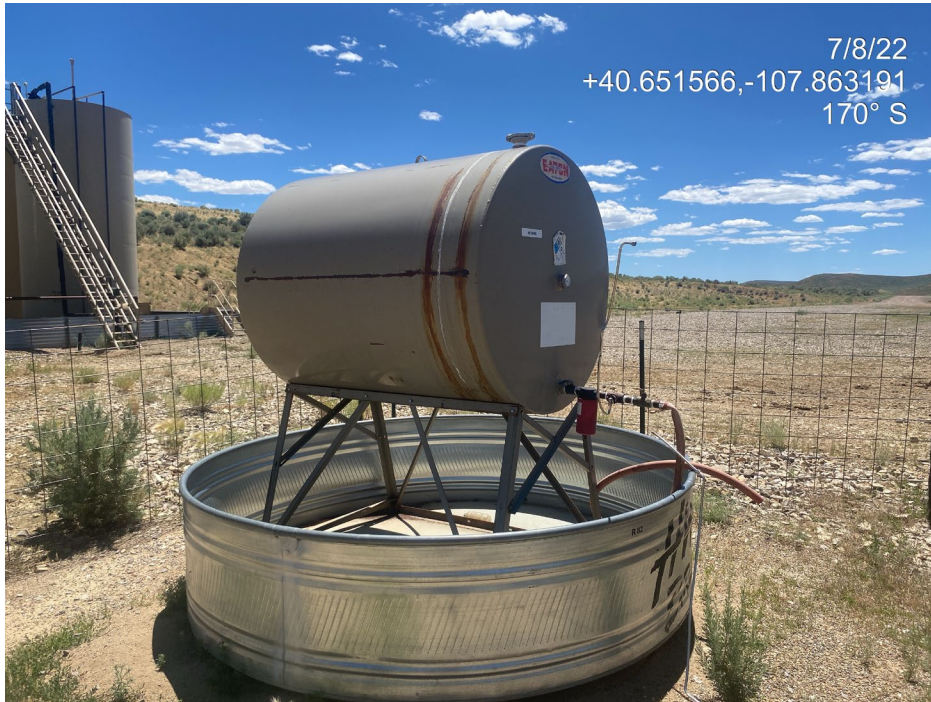
Photo 9. Photo shows a methanol tank at the north of the Location with inadequate wildlife protection BMPs on the secondary containment stock tank.
