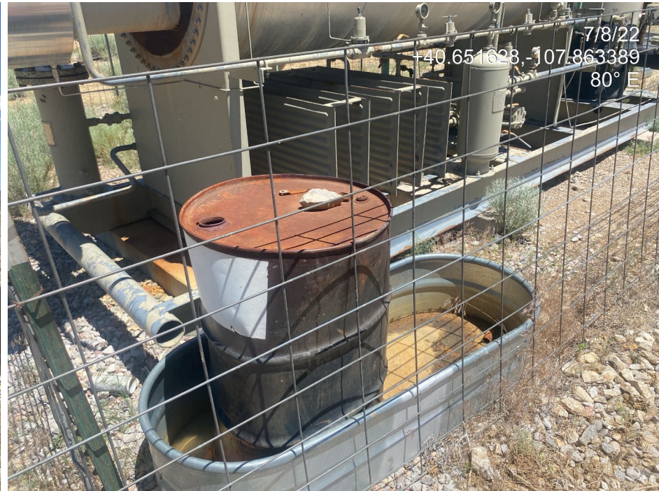
Photo 10. Photo taken at the north of the Location shows inadequate wildlife protection BMPs on the secondary containment stock tank.
