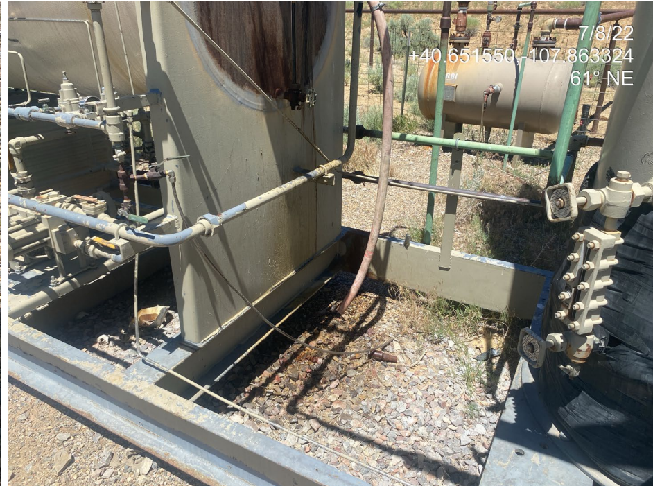
Photo 12. Photo taken at the north of the Location shows fluid dripping from separator equipment onto the ground.
