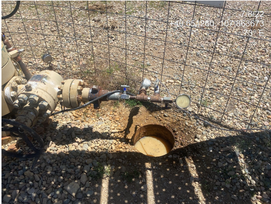
Photo 11. Photo shows an open pipe at the wellhead.
