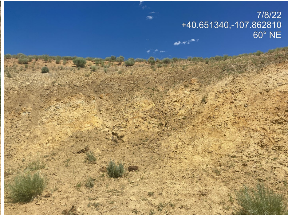
Photo 6. Photo taken from the northeast of the Location shows widespread rill erosion occurring on the cut slope.
