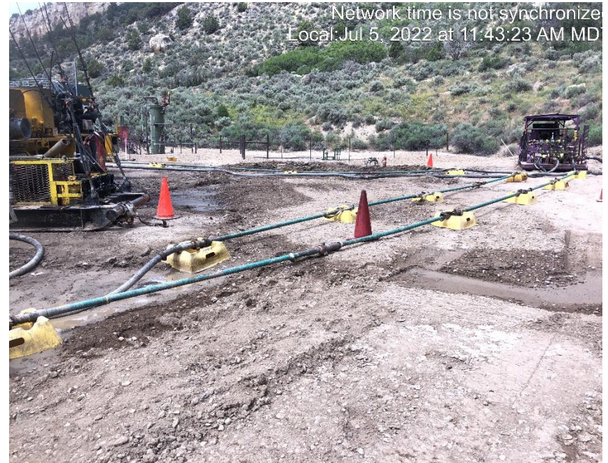
Photo #7065 The pump is now located 30 to 40 feet further from the workover rig.
