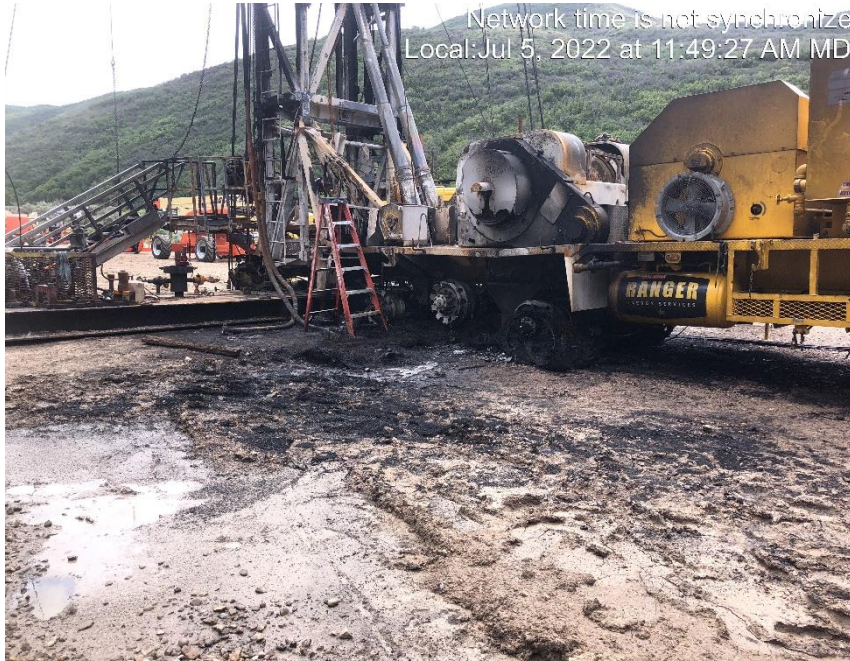
Photo #7070 Turbo side of workover rig fire.
