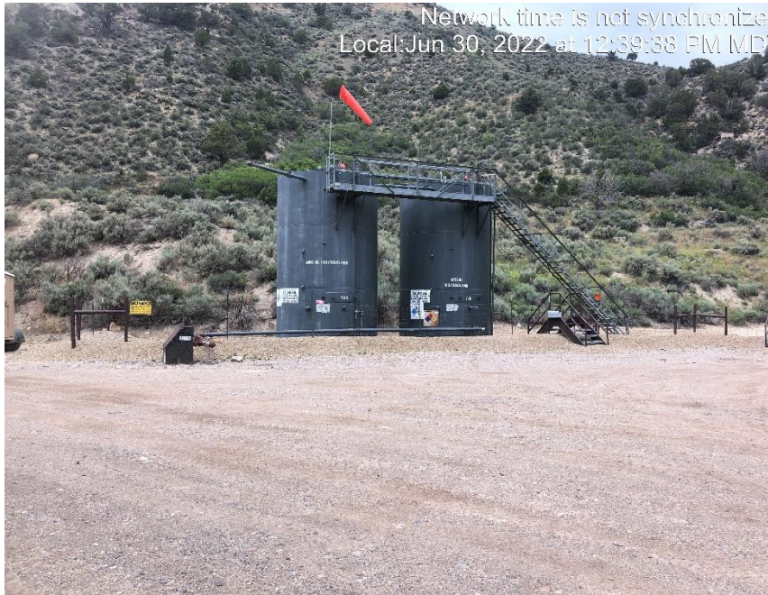
Photo #7057 Production equipment from South West side of location. Photo from inspection #699804662 conducted on 6/30/22.
