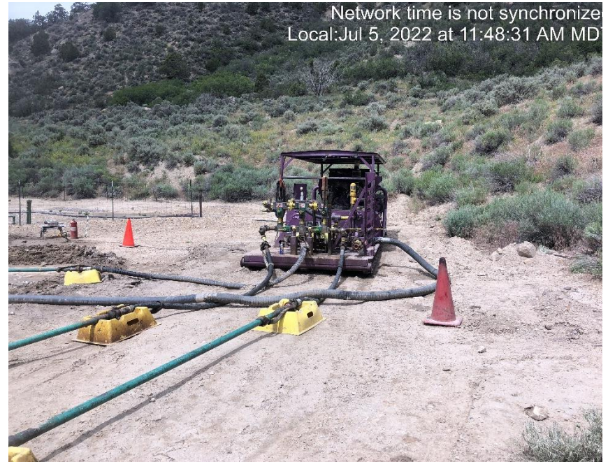
Photo #7068 New location of pump.
