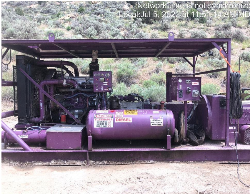
Photo #7072 Pump does not appear to have any damage from fire.
