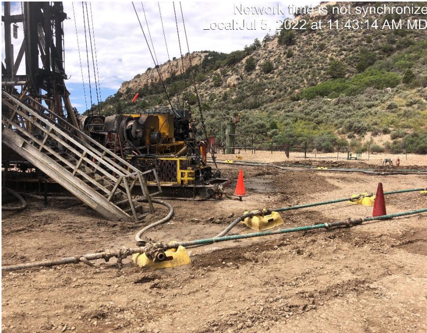
Photo #7064 The pump was located just to the right of the rig at the time of the fire which was not compliant with COGCC rules.
