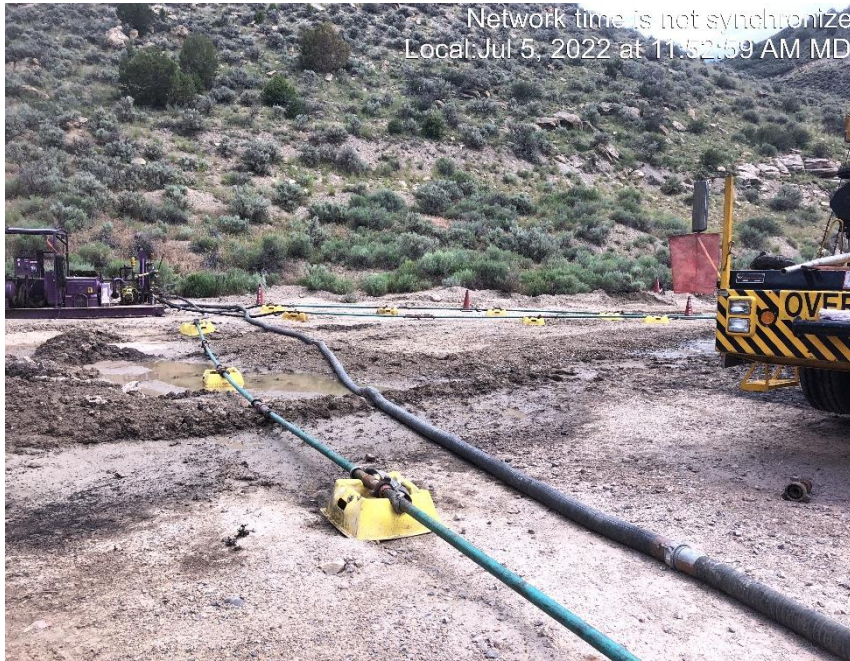
Photo #7074 New configuration of flow iron and hoses between pump and tank.
