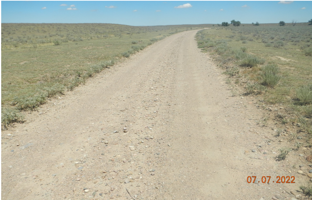
Photo 2. Facing northeast along the access road. This area along the road is stabilized with gravel.
