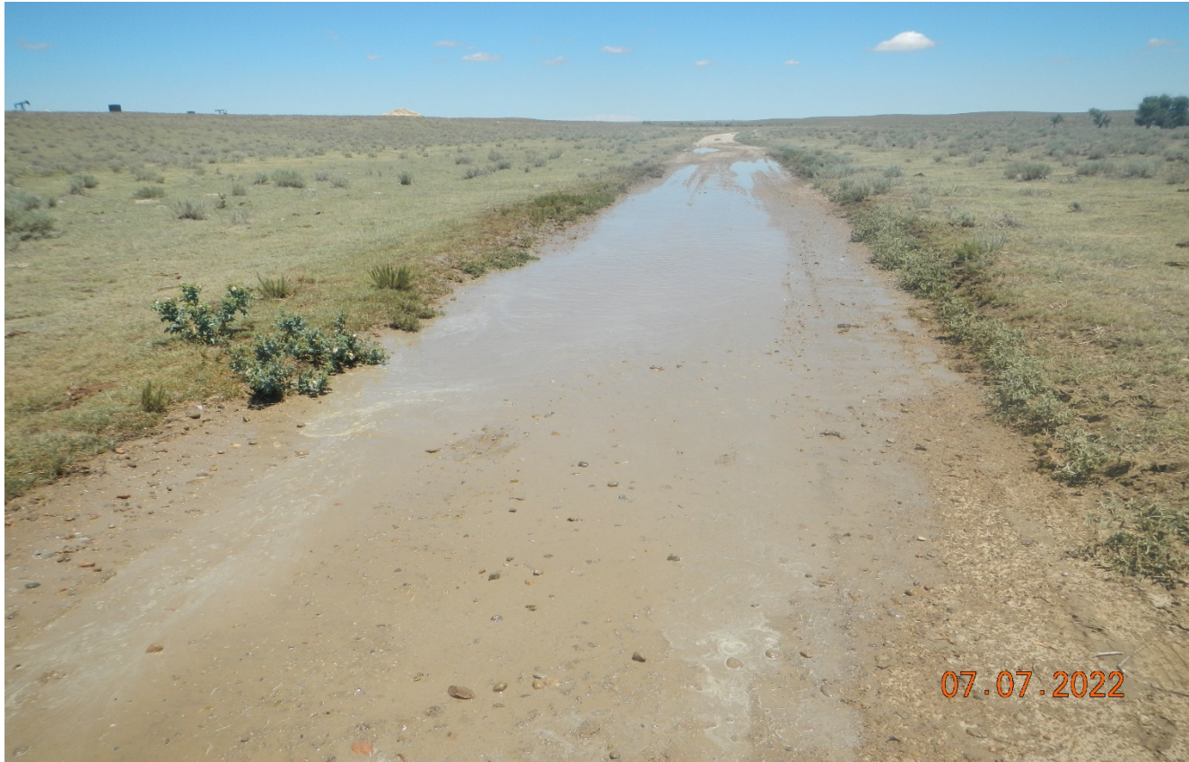
Photo 4. Facing northeast along the access road. There are areas where stormwater is pooling on the road causing vehicles to drive around and widen the road. This area needs to be stabilized with BMP's such as gravel. Stormwater should be diverted off the road.
