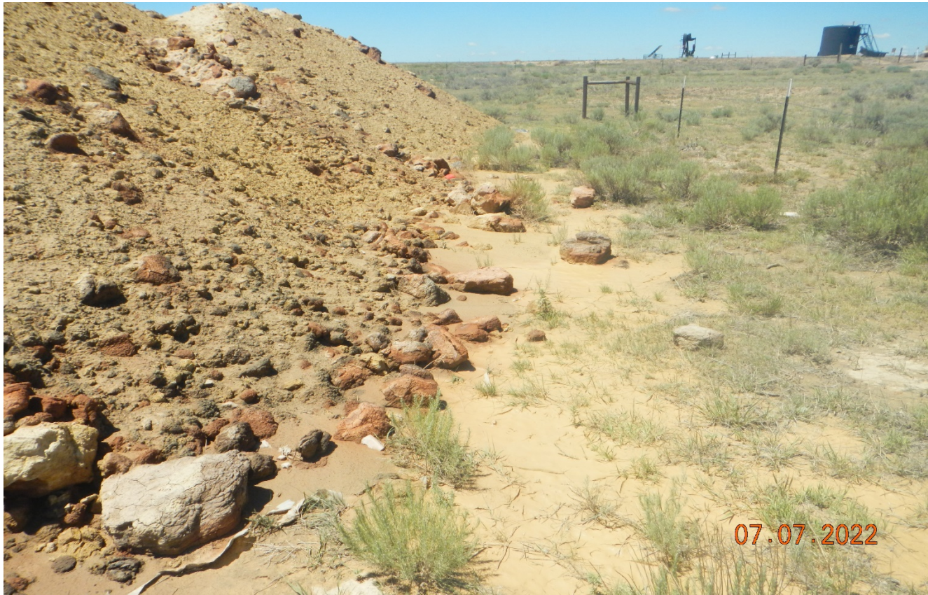
Photo 13. Facing west toward the excavated material stored onsite. There are no perimeter BMP's around the excavated material to prevent sediment transport offsite. There are signs this material has eroded offsite from recent precipitation.
