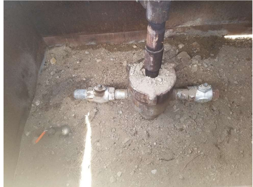
Photo 2. Photo of wellhead inside housing cover.
