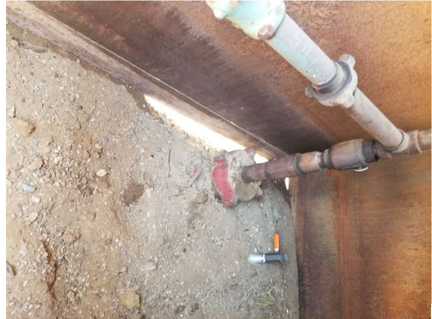
Photo 2. Photo of wellhead inside housing cover.
