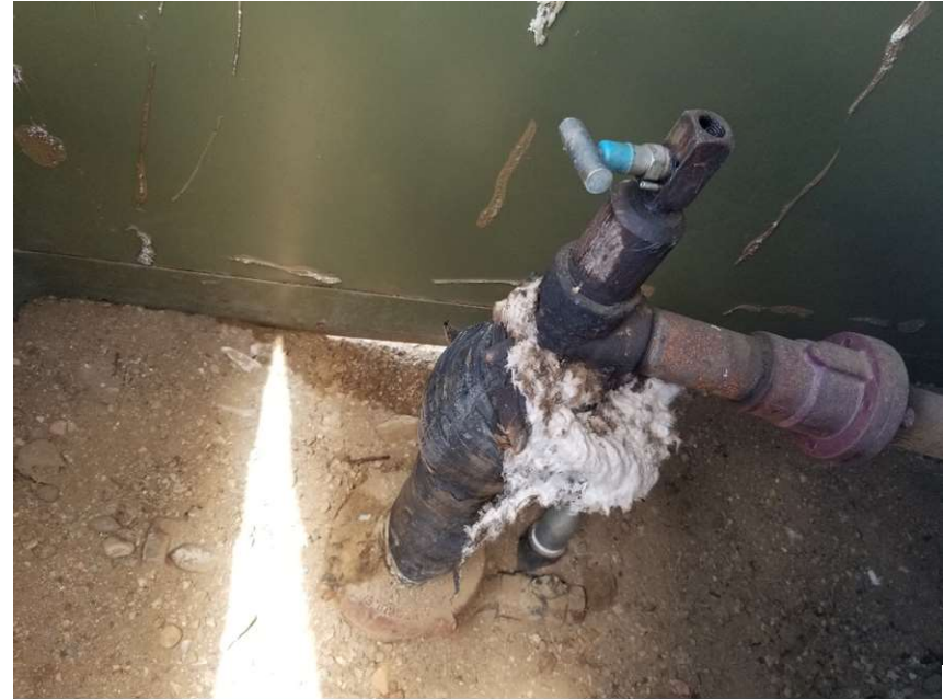
Photo 2. Photo of wellhead inside housing cover.
