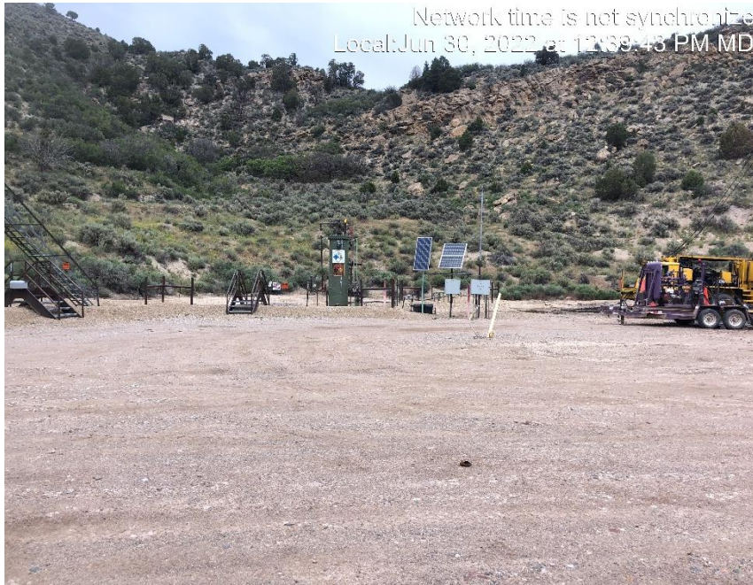
Photo #7058 Workover rig and tank battery stair case.
