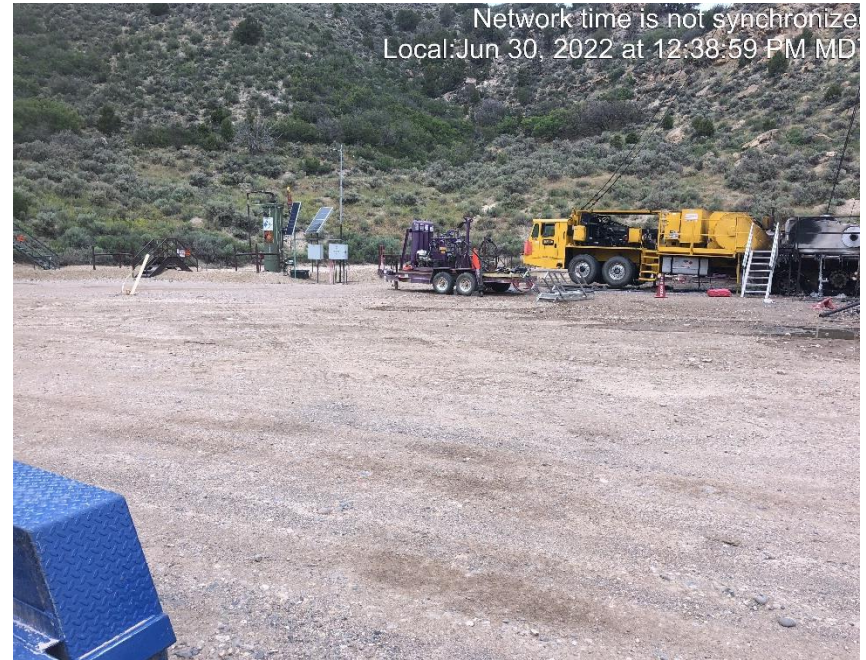
Photo #7056 Nearest production equipment to workover rig and accumulator.
