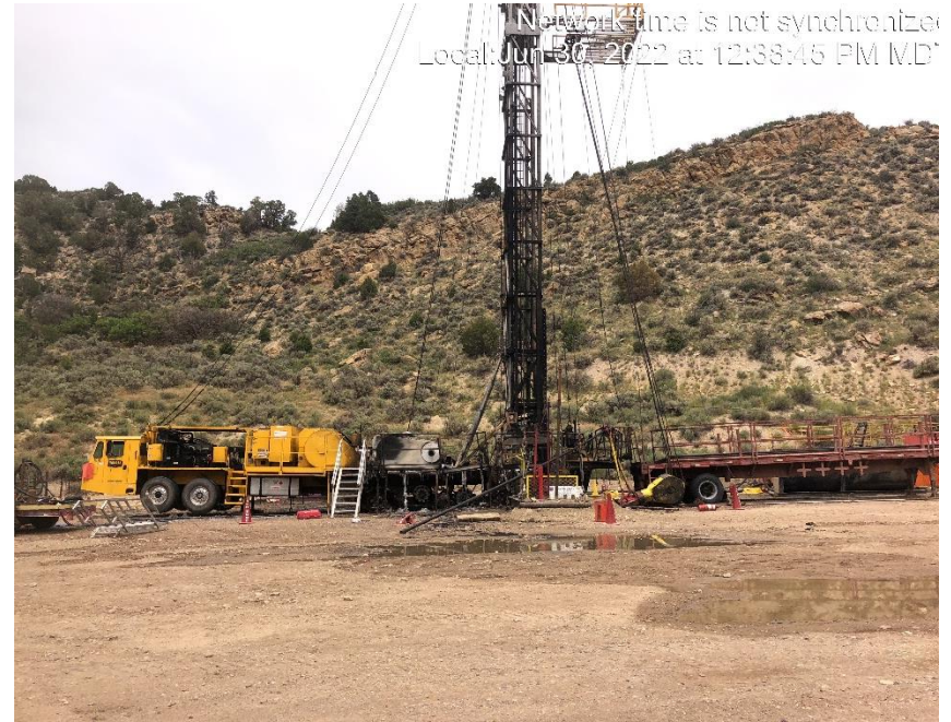
Photo #7054 Workover rig fire.
