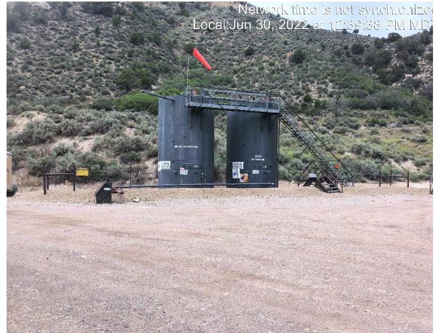
Photo #7057 Tank battery.
