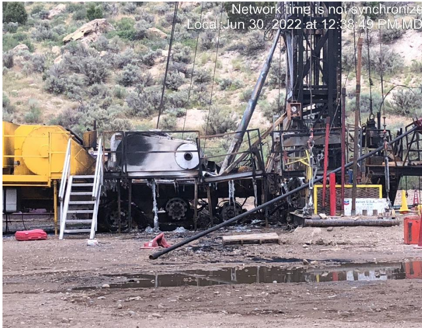
Photo #7055 Workover rig fire.
