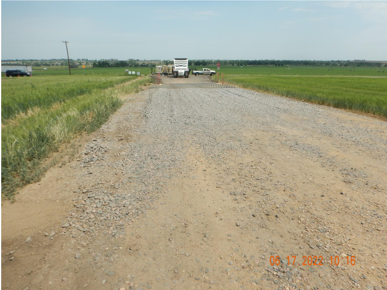
Photo 3. Photo taken south of the entrance, facing North. Photo illustrates additional tracking device BMPs have been added (additional rock, recycled asphalt and additional roadbase was added to the entire access road). Also, Operator performed the required BMP maintenance.
