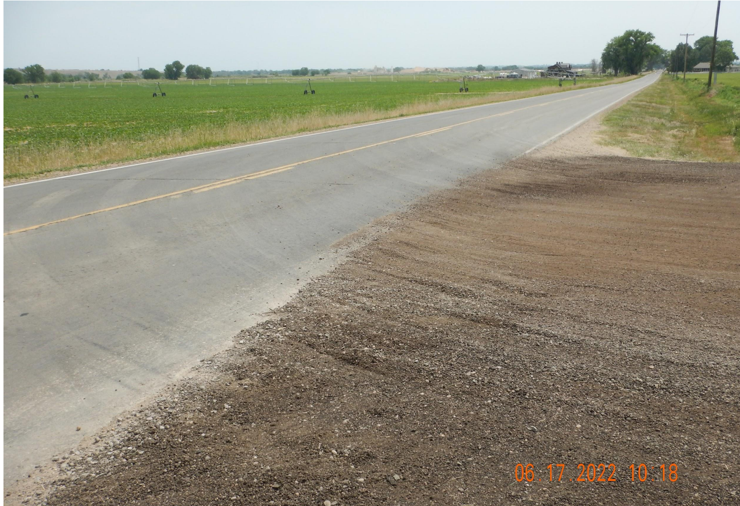
Photo 1. Photo taken from the entrance of location, facing East. Photo illustrates Operator has cleaned up the sediment track out and there were no observed issues during this inspection.
