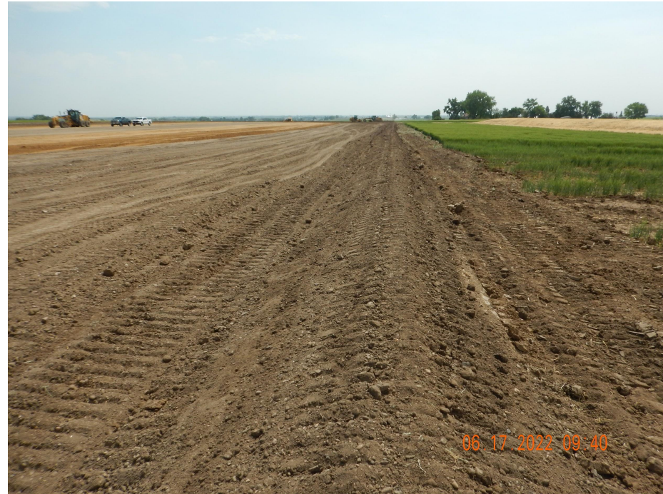
Photo 5. Photo taken from the southwestern well location, facing East. Photo illustrates a graveled berm BMP has been installed as an additional stormwater BMP.
