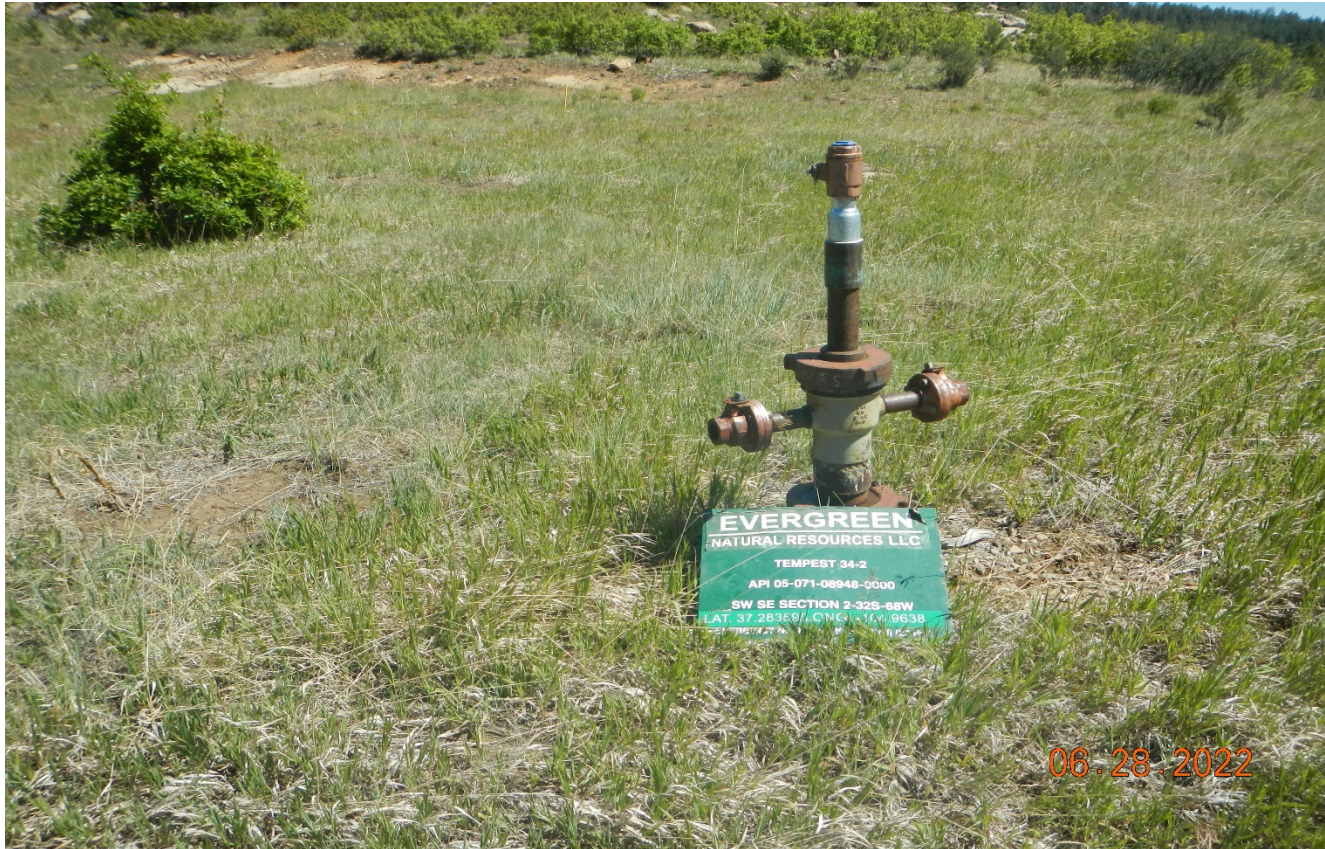
Photo 2. There is a sign at the wellhead but it is not securely installed.
