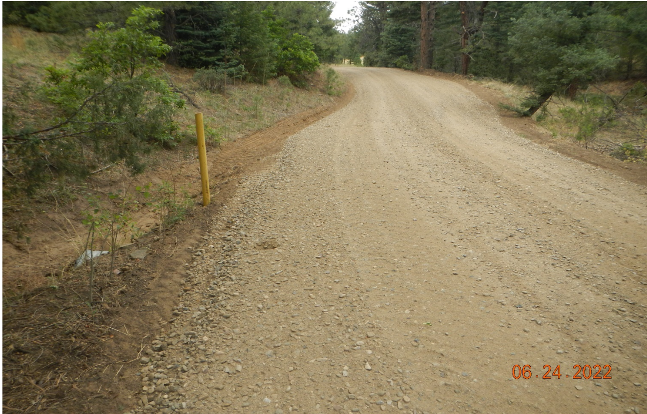
Photo 1. Facing west along the main access road. There has been additional gravel spread along the road and the culverts are maintained.
