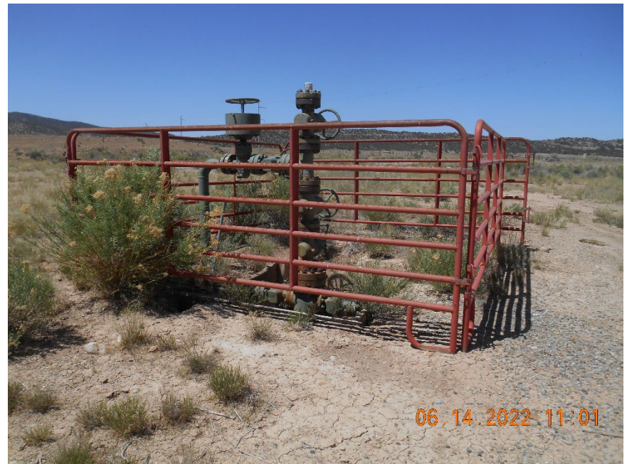
Wellhead with fencing
