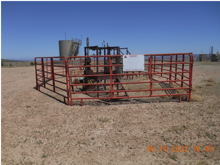
Wellheads with fence and signs
