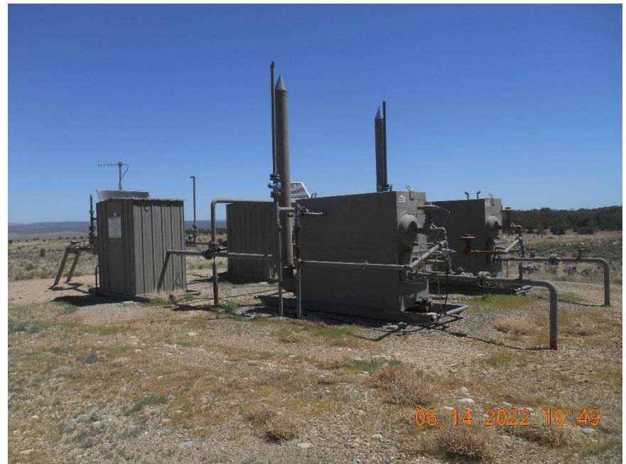
Separators and Meter housings
