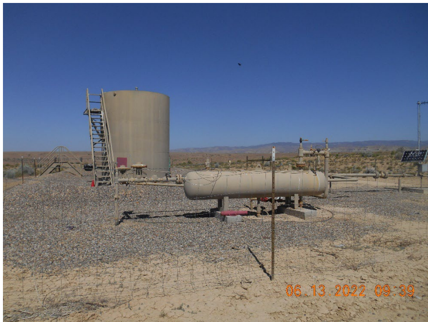
Separator and meter
