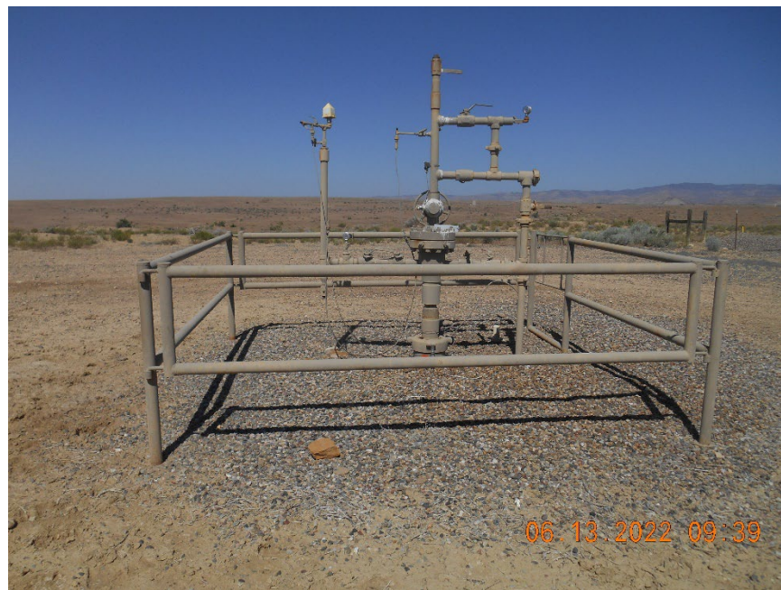
Wellhead with fence
