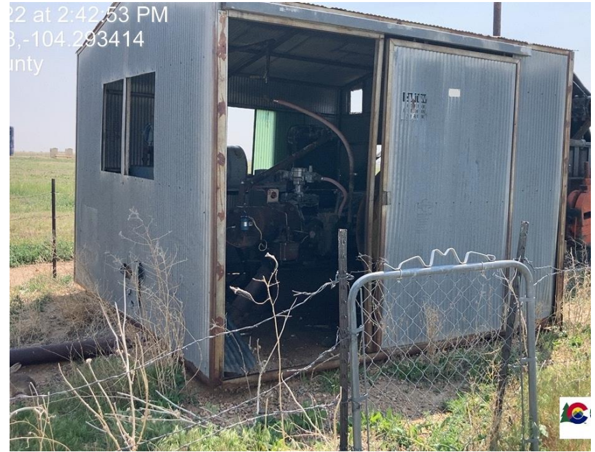
Pic 4 stained soil in motor house
