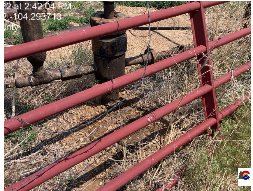
Pic 2 bradenhead is not plumbed to surface, stained soil
