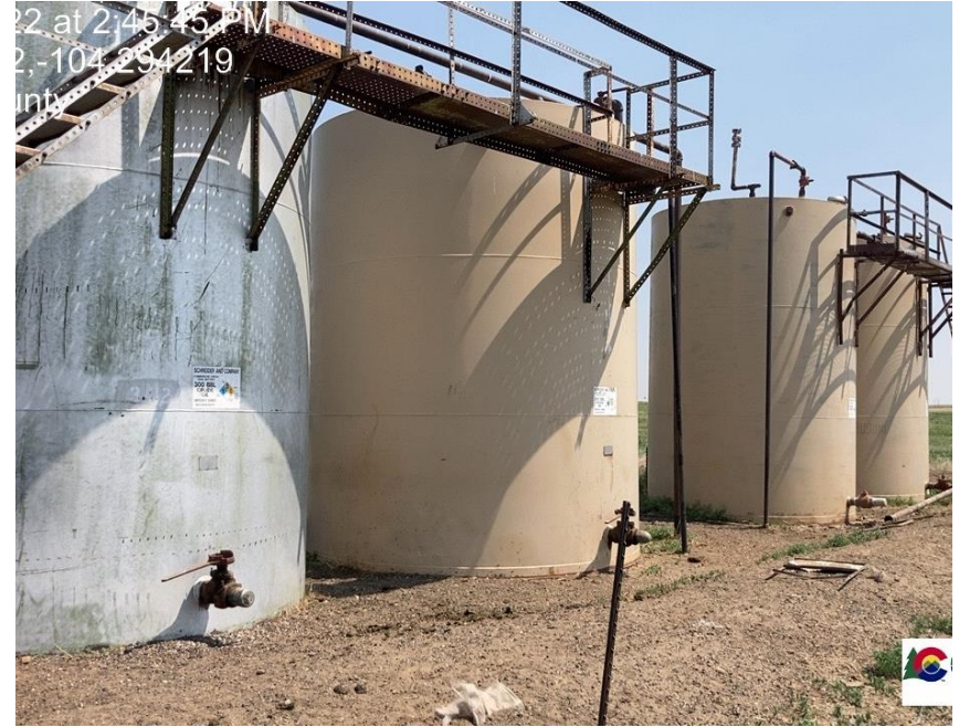
Pic 6 tanks berm is inadequate
