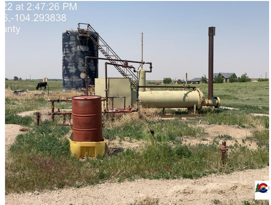
Pic 8 unused equipment / risers, separator
