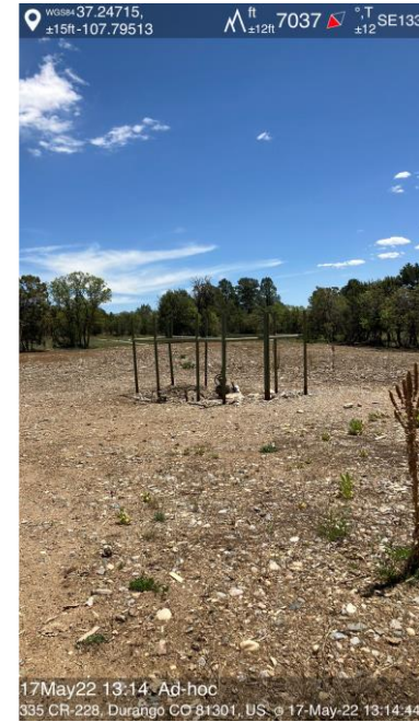
IMG 04 Wellhead with protective barriers
