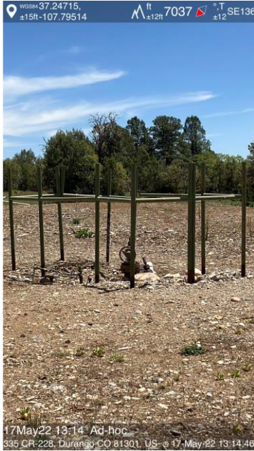
IMG 05 Wellhead with protective barriers
