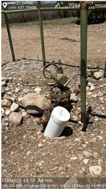
IMG 09 Wellhead with accessible bradenhead
