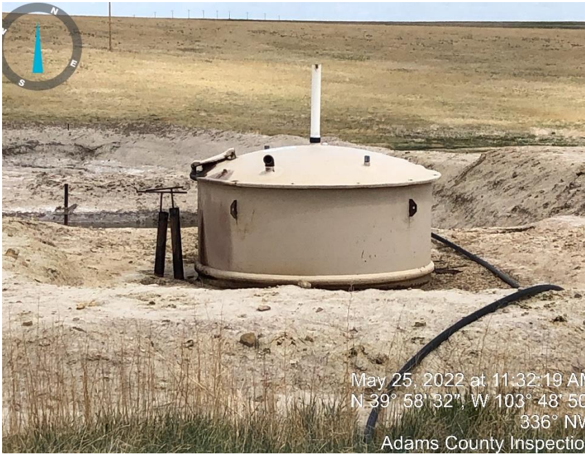
Photo #3 Produced water tank.
