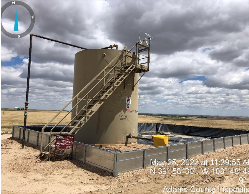
Photo #1 Crude tank.
