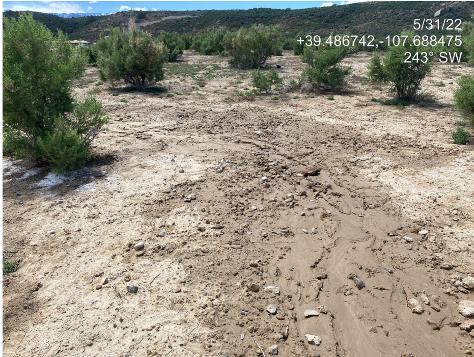
Photo 5. Photo taken from the north of the Location shows where a gully was raked. Erosion continues at the site, as no control measures were implemented to stabilize soils.
