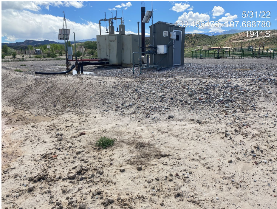
Photo 1. Photo taken from the east of the Location behind the separator shows the previously undermining berm is intact. Photo shows the view from the outside of the berm.
