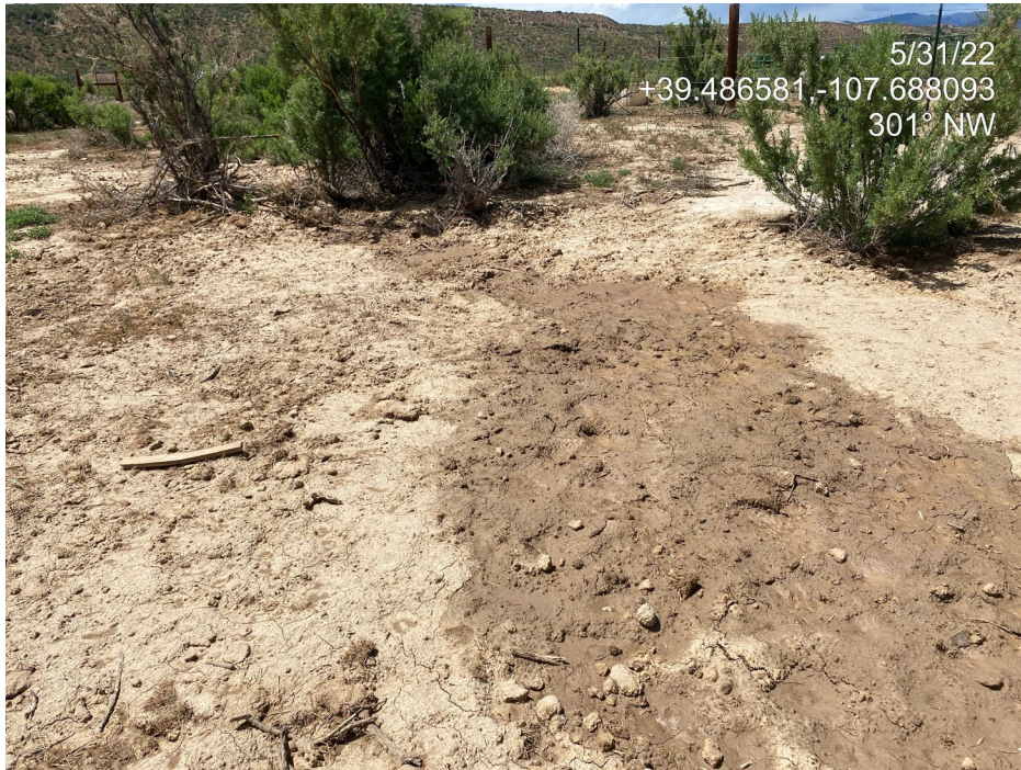
Photo 3. Photo taken from the east of the Location shows where erosion was raked. Erosion continues at the site, as no control measures were implemented to stabilize soils.
