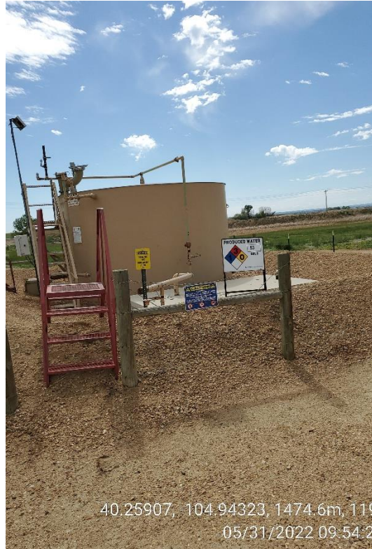
Photo 2 Battery with Produced Water Capacity Sign
