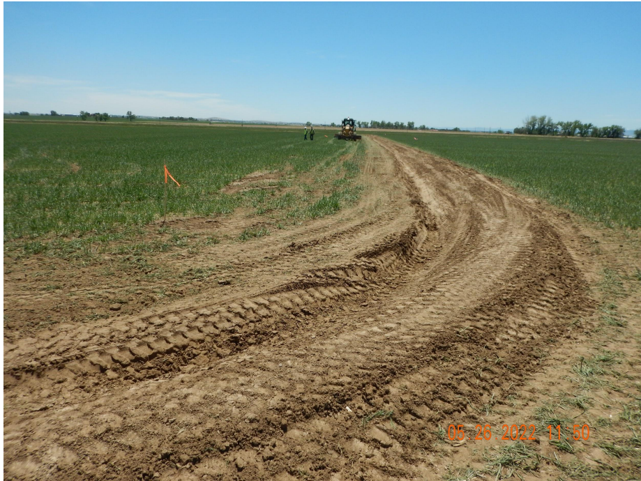
Photo 5. Photo taken from the northwestern location, facing South. Photo illustrates a ditch and berm BMP that has been installed around the entire perimeter of location.
