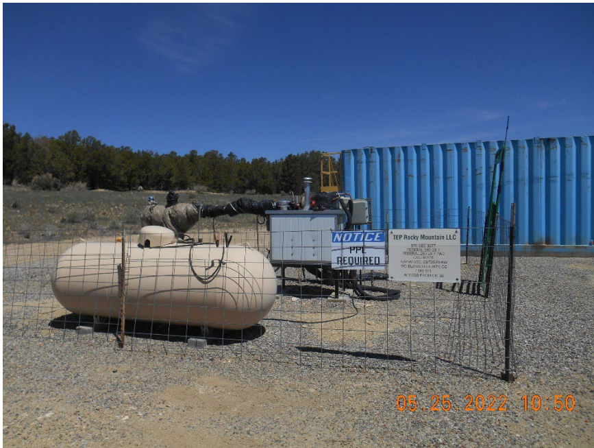
Injection wellhead & line heater
